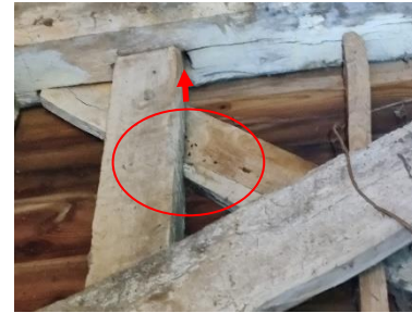
Natterer's bat droppings (confirmed by eDNA analysis) found below vertical opening in joint on western wall of barn during building inspection
