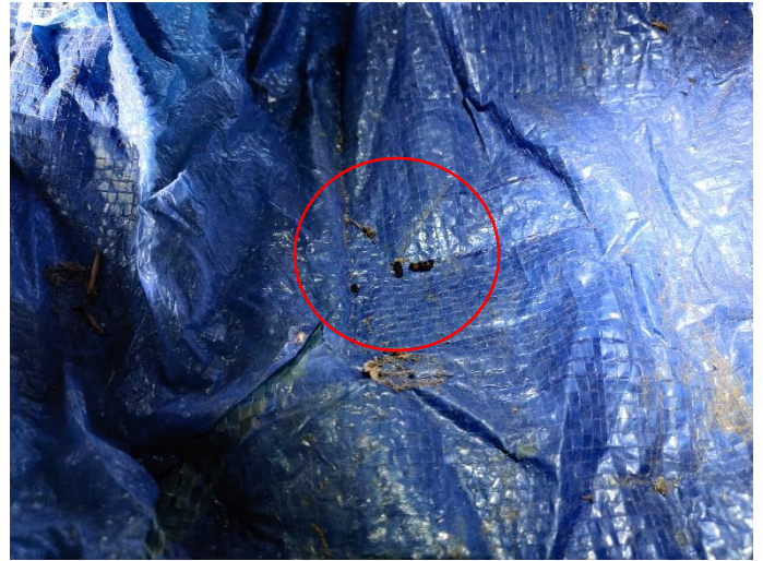
Photo 14 Bat droppings on plastic tarpaulin below roost location on west wall
