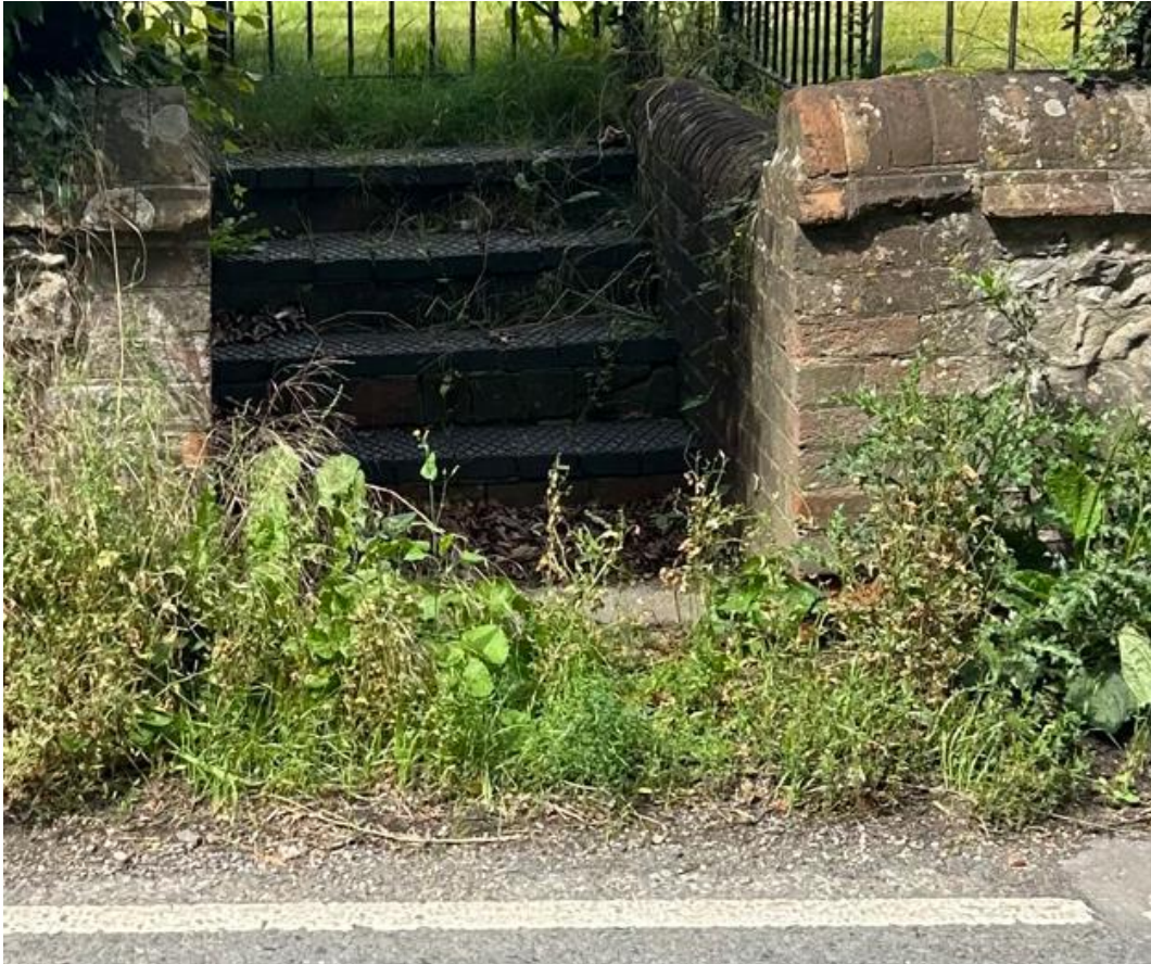
Photo 12: Close-up of the flint wall on the B3400
