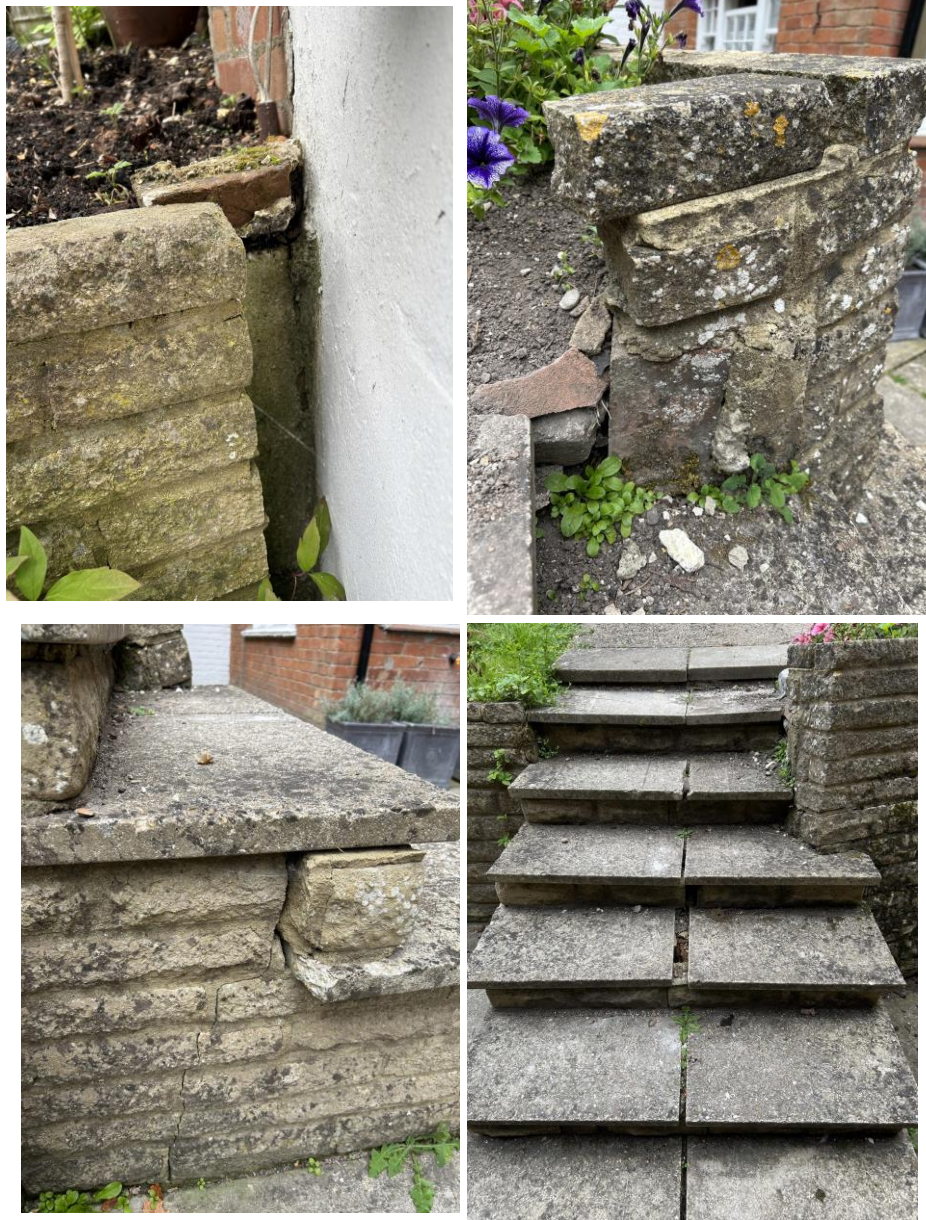
Photos 24 – 26: Poor construction
