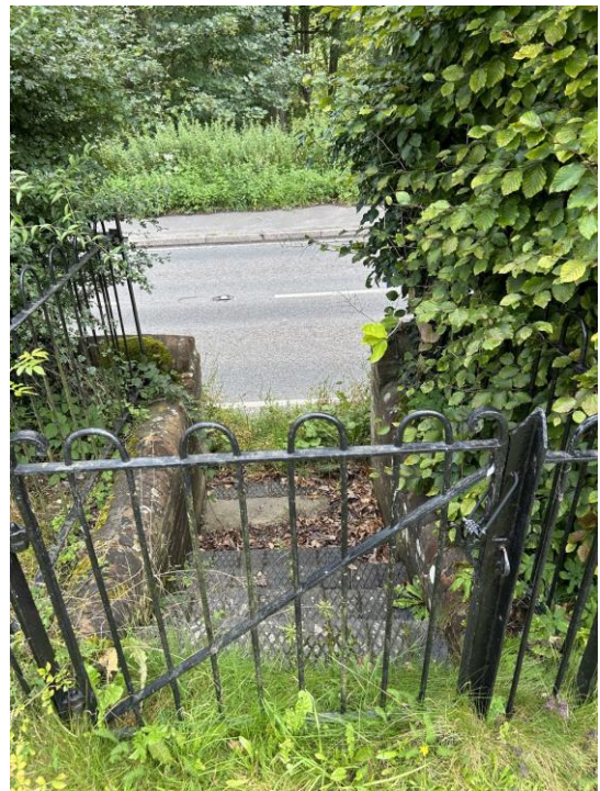
Photo 10: Close-up of metal gate and railings on the B3400 (padlocked for safety)
