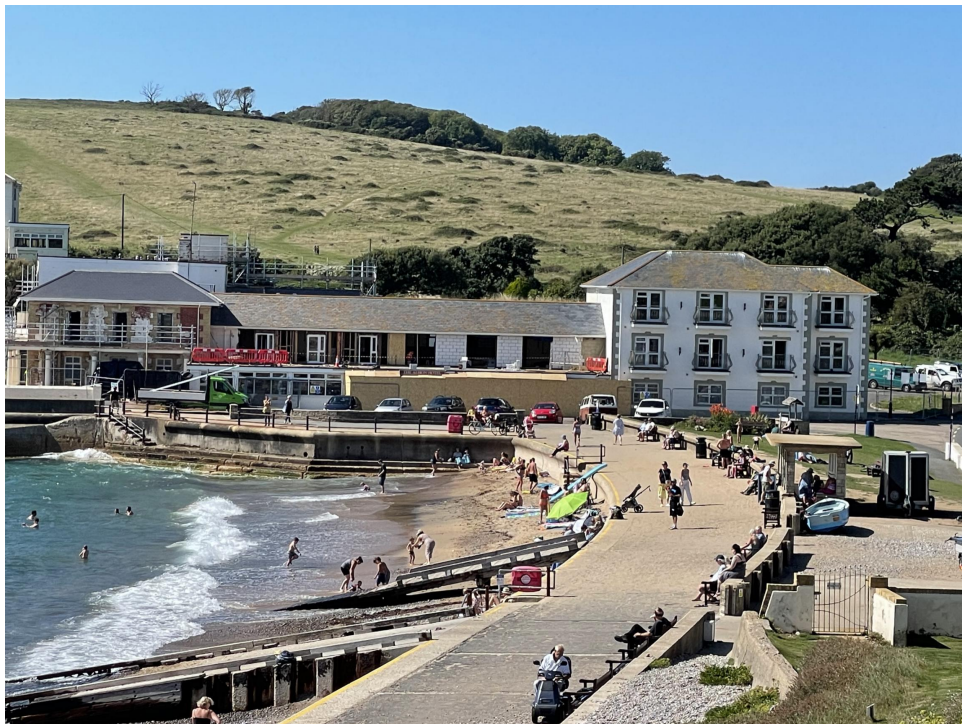
The Albion Hotel. A very prominent building undergoing refurbishment at present with a substantial increase in the glazing. A good design taking advantage of the wonderful sea views.
