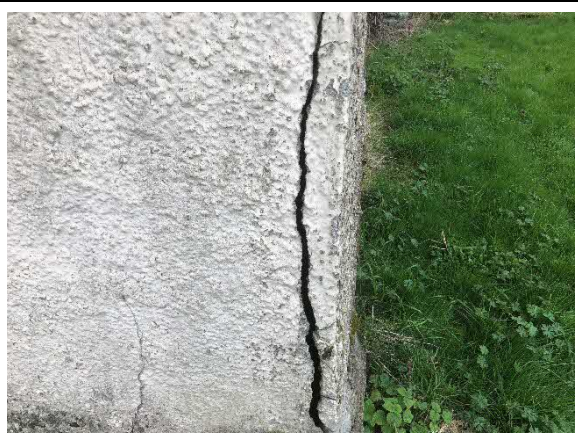
Cracks to walls at ground level.
