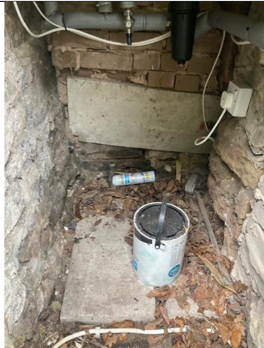
Plate 8 – location of pipistrelle sp, dropping on floor of boiler room
