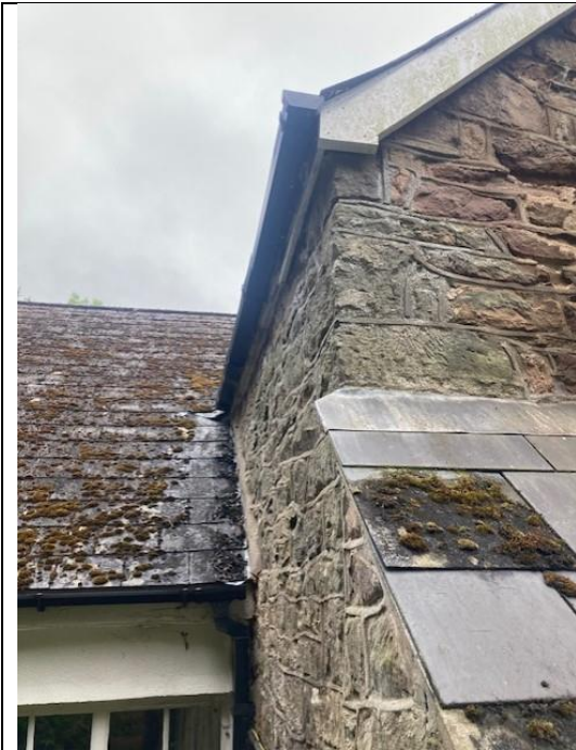
Plate 5 – fascia boards on northeast and north west elevations of cottage showing section of rot on northeast elevation
