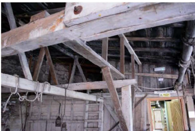
Photo 3. Main void in bagging shed (with shop to rear), viewed from NE.
