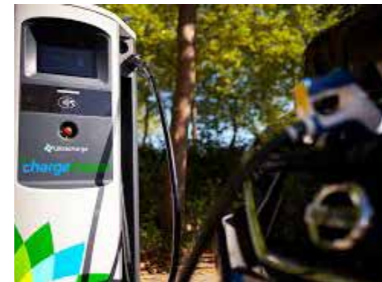
Electric charging points
