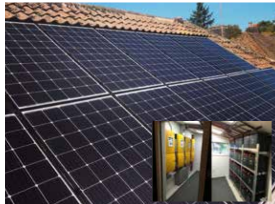
Photovoltaic cells & battery storage
