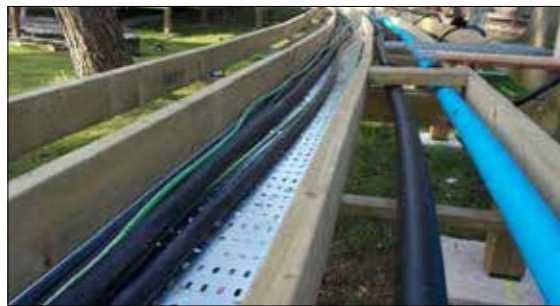
MAIN SERVICES CONTAINED IN BOARDWALK
