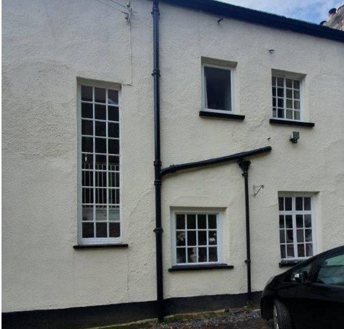
Photo above showing patchy/ deteriorating cement render
