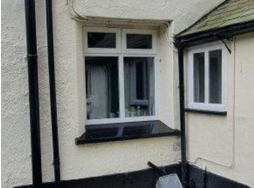
Photo above showing W4.
