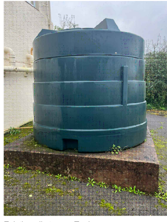
Existing oil storage Tank
