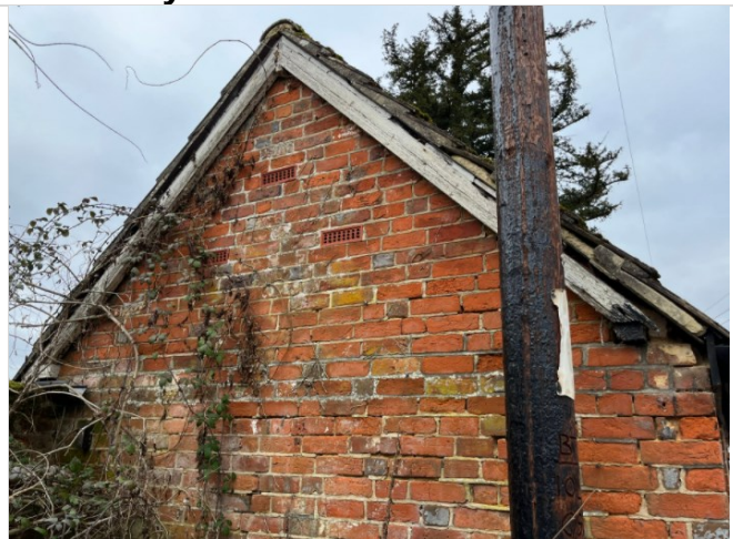
Gaps at dry verges
