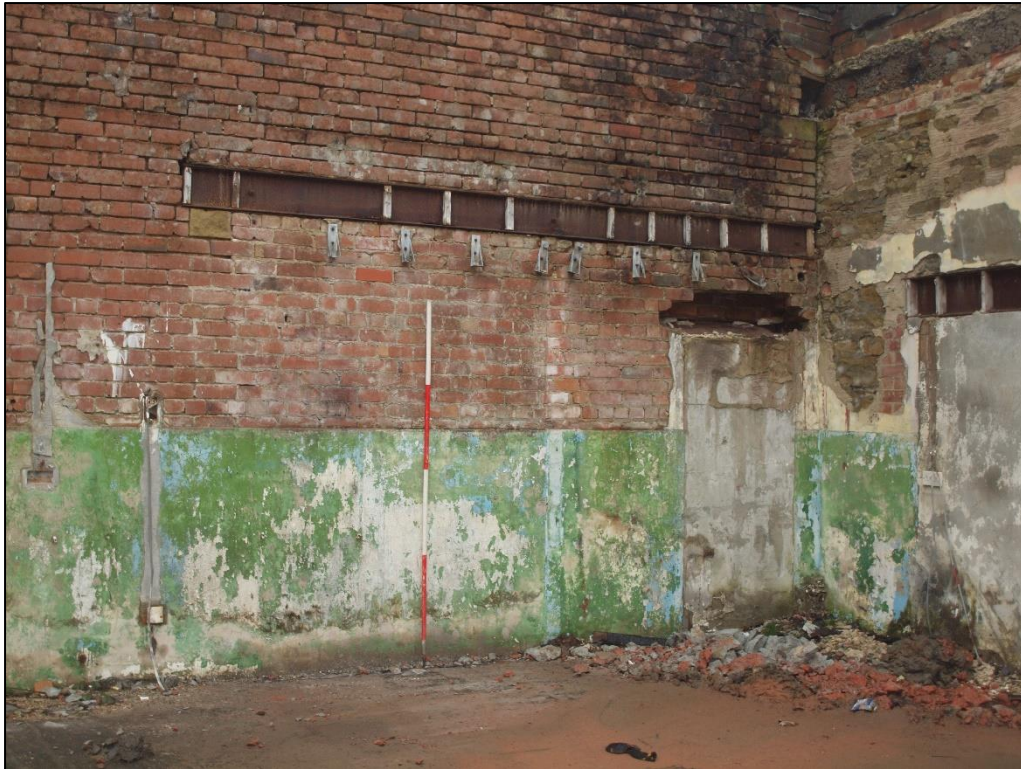
Plate 37: Blocked doorway to east side, with large lintel over showing location of former loading doorway
