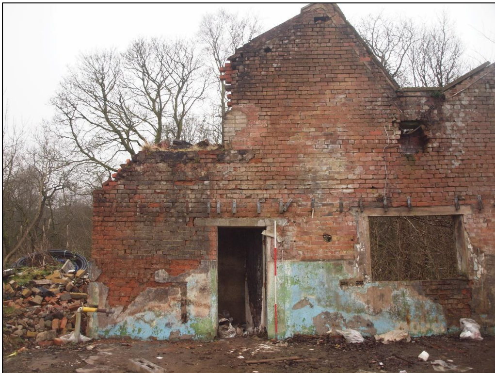
Plate 24: East end showing damaged gable
