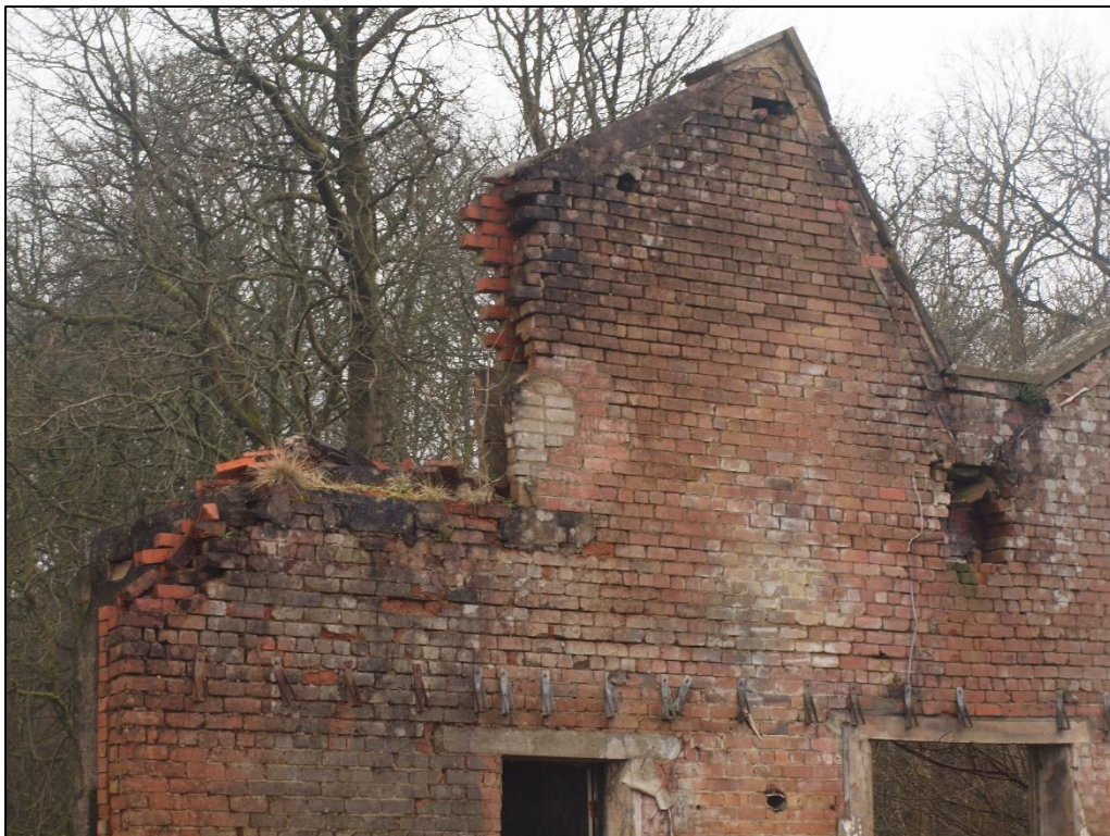
Plate 26: Gable showing damaged blocked opening
