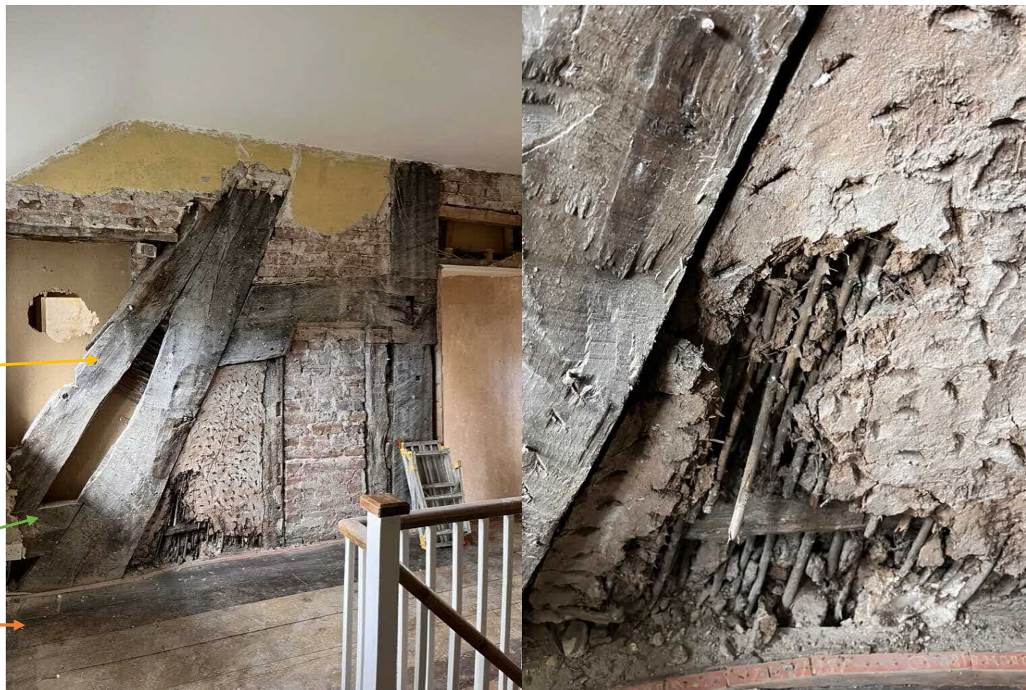
Fig 9. The cruck to first floor above the screens partition showing wattle and daub and later brick infill. Note the packing piece (arrowed yellow) and the spur (arrowed green). The tie beam (arrowed orange) at floorboard level appears original to the truss.
