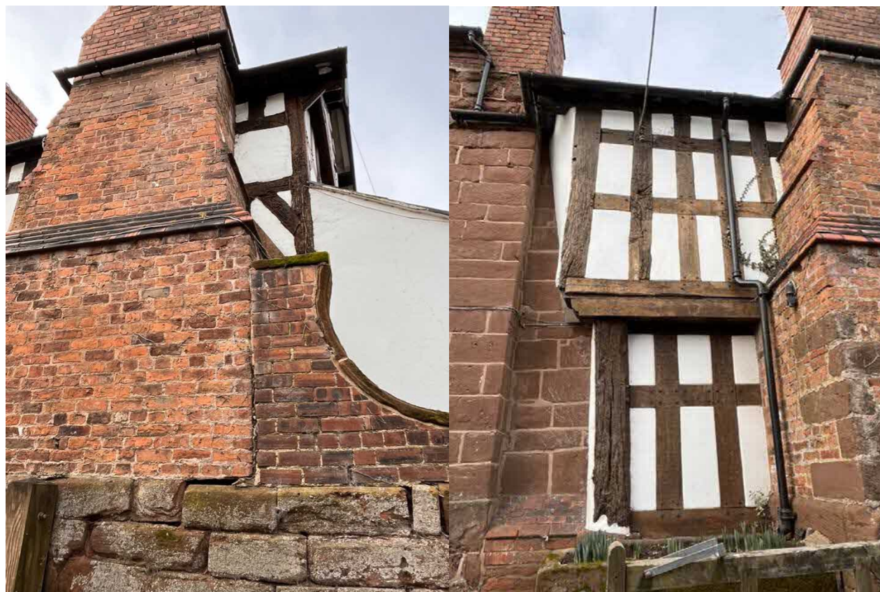
Fig 5. The east elevation of Churton Hall, 2023. Note the curved wall adjacent to the lateral chimney stack shown in the image of 1793. The second photograph shows the jettied first floor and close studded timber framing, truncated by a coursed sandstone wall, part of the second lateral chimney stack – the earlier one is of stone.
