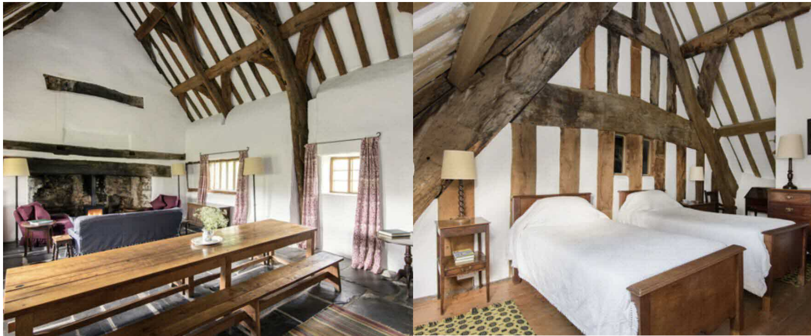
Fig 16. Left: Plas Uchaf, near Corwen, Denbighshire, a hall house of c1400. (Grade I)
