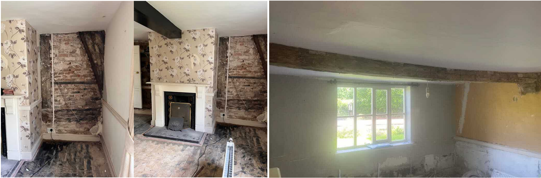
Fig 8. The other side of the screen passage inserted next to an early 20 th century fireplace. The floorboards were probably installed at the same time, or later. The sandstone cellar is underneath this floor. A stop chamfered beam is encased in plaster and painted black gloss. This has now been uncovered. It has been raised and is resting on a corbel that may indicate the location of the division wall between pantry and buttery.
