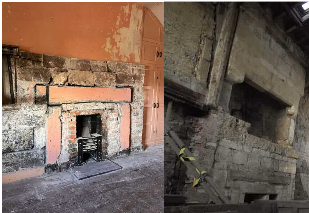
Fig 14. The fireplace to the solar, or chamber above the east room with inglenook. Note the various changes to the fireplace as flues became slimmer. The sandstone blocks are substantial. The Georgian grate was probably inserted in the early 19 th century with other improvements undertaken at the time. The image to the right is that of Llwyn Celyn, a late medieval hall house of 1420. Note the similarities of the ground floor fireplace to that at Churton.
