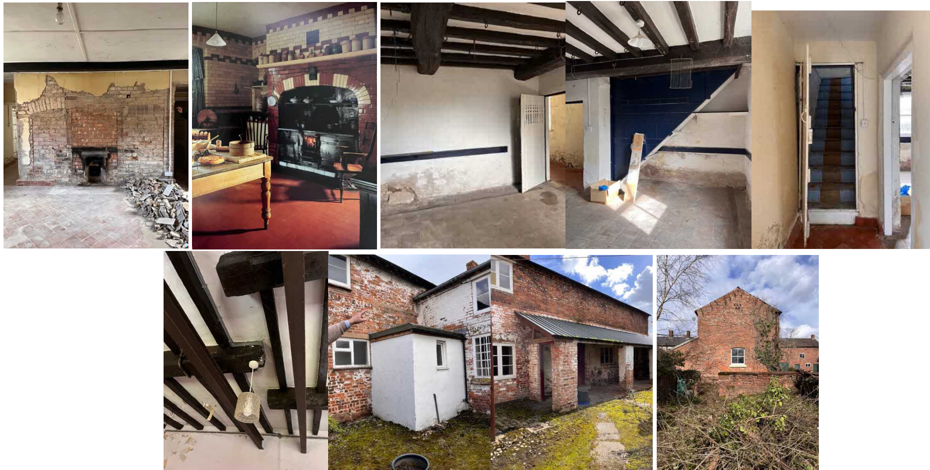
Fig 22. Features of the Victorian wing including from top left to right: the former kitchen range area – the second image is from ‘The Victorian Society Book of the Victorian House’, image 3 and 4 show the meat room and the later staircase to be removed, which will reinstate the room proportions. Bottom left to right; evidence of a missing wall to be reinstated, the flat roofed modern WC behind main house; the functional veranda to be removed – former dairy area; and the south facing gable.
