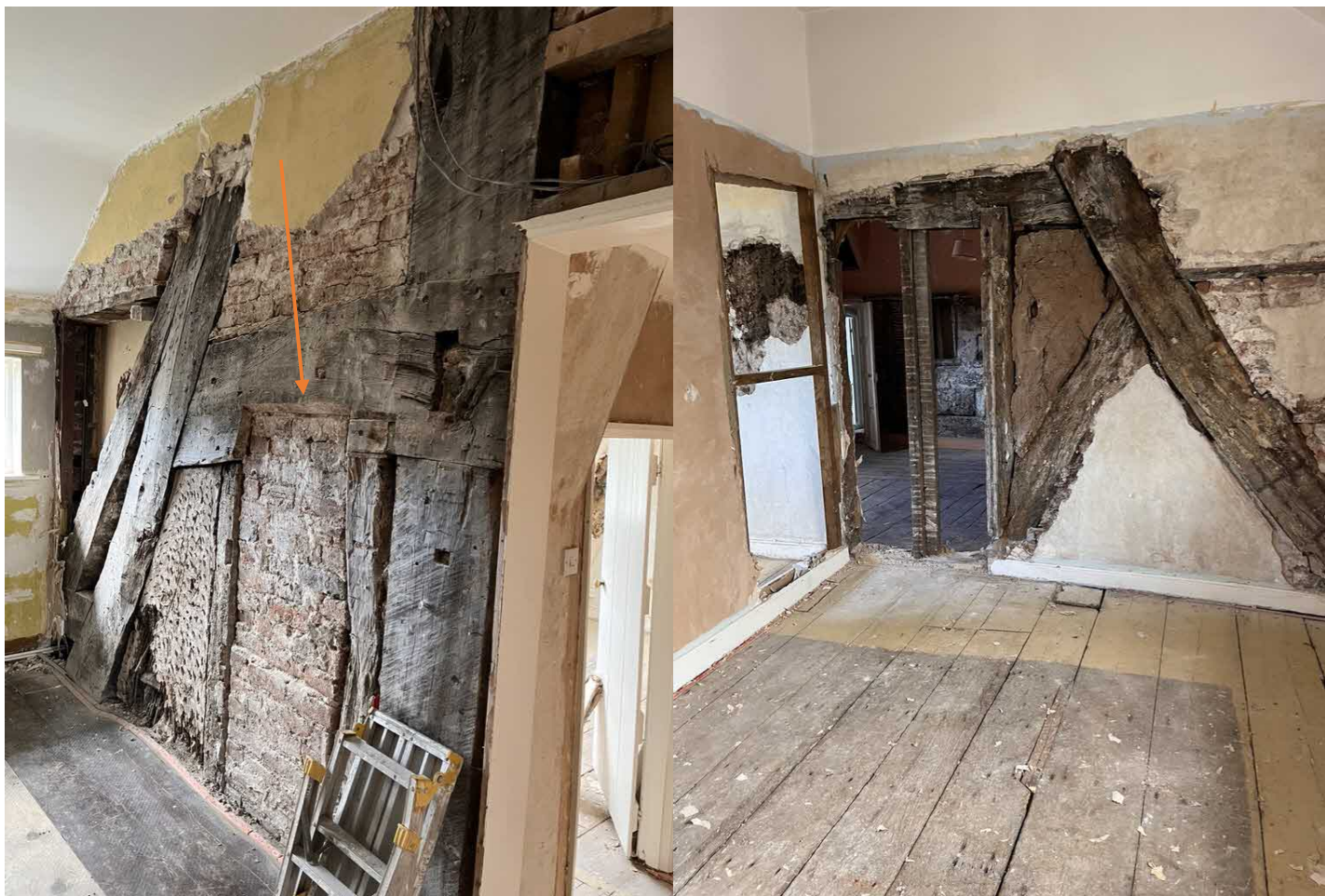
Fig 10 The crucks to first floor. To the left is the cruck above the screens partition. Note the inserted door (arrowed orange). To the right is between the 17 th century chamber with lateral chimney and inner room. Note wide floorboards.
