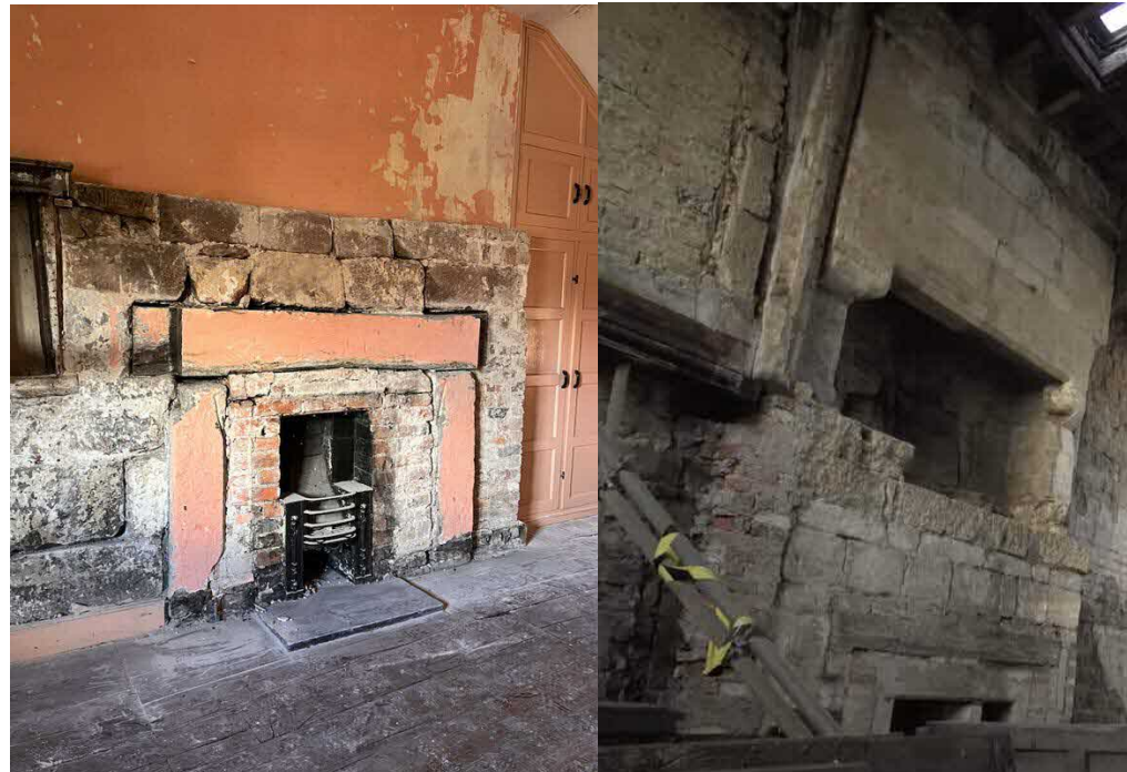
Fig 14. The fireplace to the solar, or chamber above the east room with inglenook. Note the various changes to the fireplace as flues became slimmer. The sandstone blocks are substantial. The Georgian grate was probably inserted in the early 19 th century with other improvements undertaken at the time. The image to the right is that of Llwyn Celyn, a late medieval hall house of 1420. Note the similarities of the ground floor fireplace to that at Churton.
