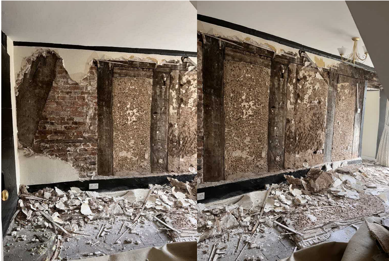
Fig 7. The assumed screens partition within the cross passage. Note the cruck to the left of the first photograph.
