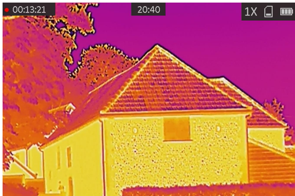
Plate 1 - Lynx Pro LH Thermal Imaging camera covering the NE elevation.
