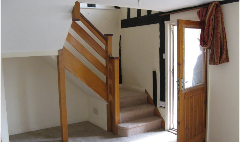
Staircase to be reorientated and replaced (No. 93).
