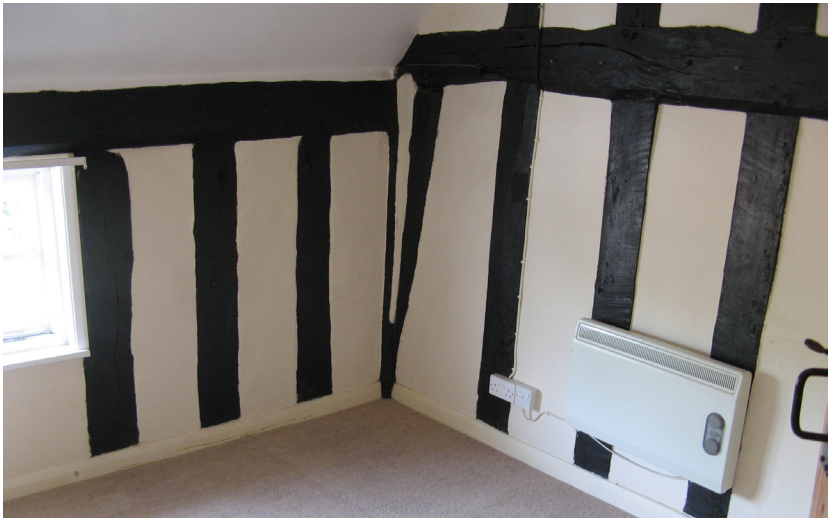
Typical quality of the timber frame as expose on the first floor.
