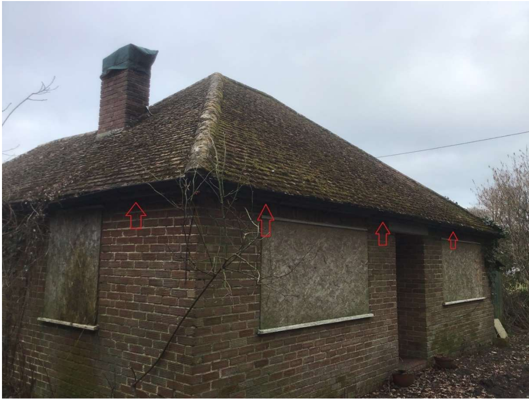
Figure 4. Western and southern elevations looking northeast. Red arrows indicate potential access points for roosting bats,
