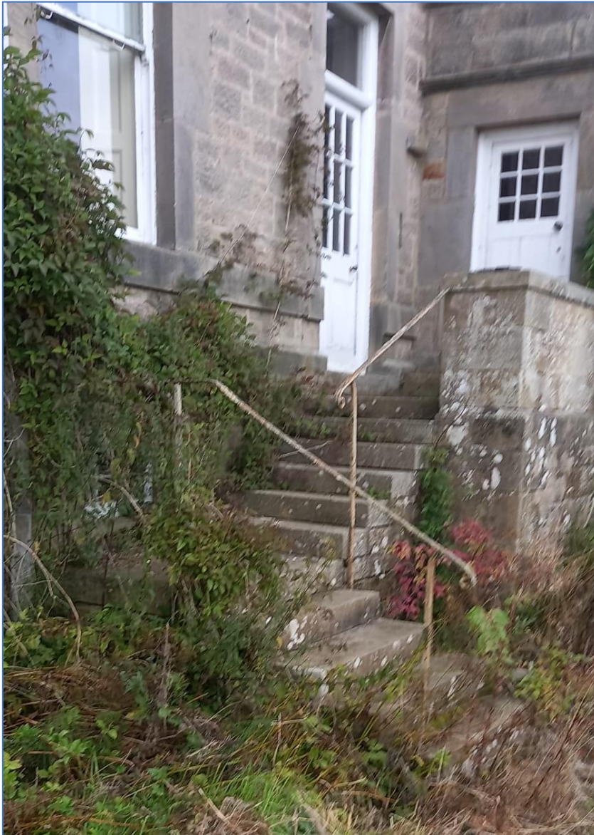
Staircase on East Elevation to be repointed & handrail replaced
