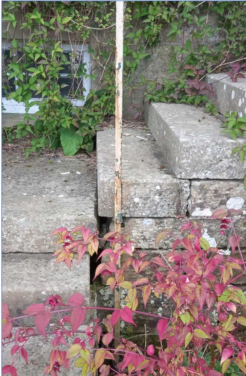
Staircase on East Elevation to be repointed & handrail replaced
