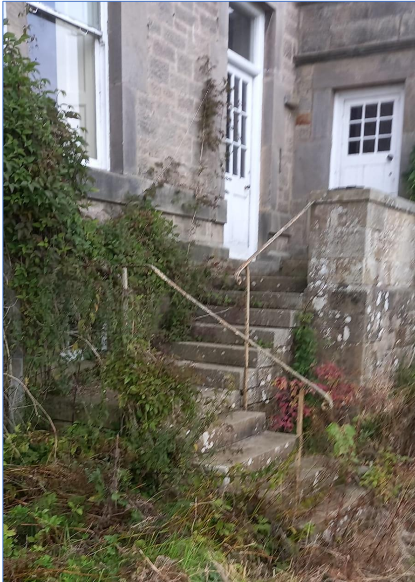
Steps on East elevation to be repaired & handrail replaced
