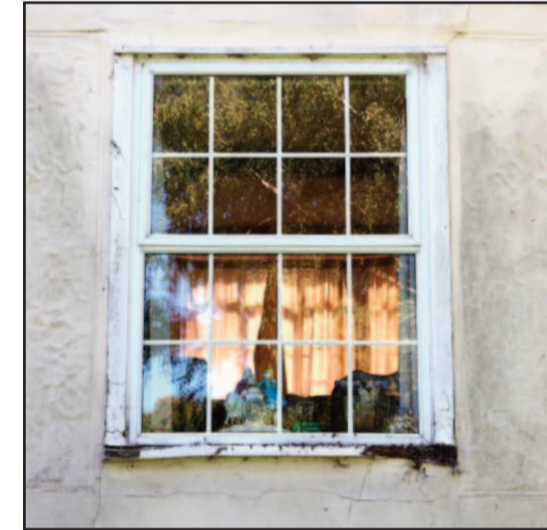
Rotting timber cills and timber surrounding aluminium windows
