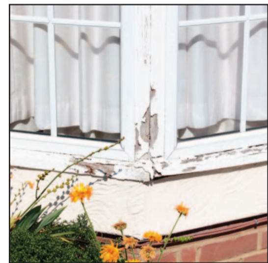
Timber bay frame requiring attention.
