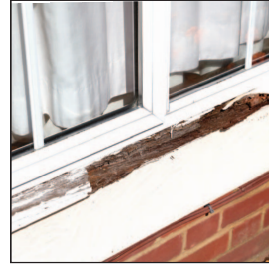
Rotting timber cills
