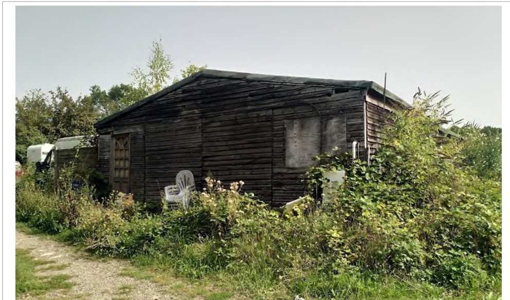
Image 6: Large storage building. This building is actively used for storage purposes. This building did not form part of planning application 22/00281/FULL. As such, it is a retained building.
