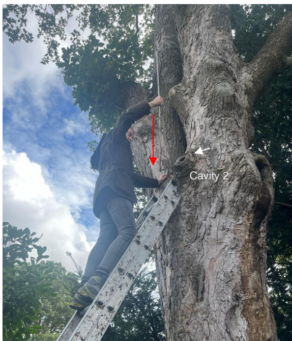
Photograph 3 – T1, cavity 2 and how far it extends into the tree
