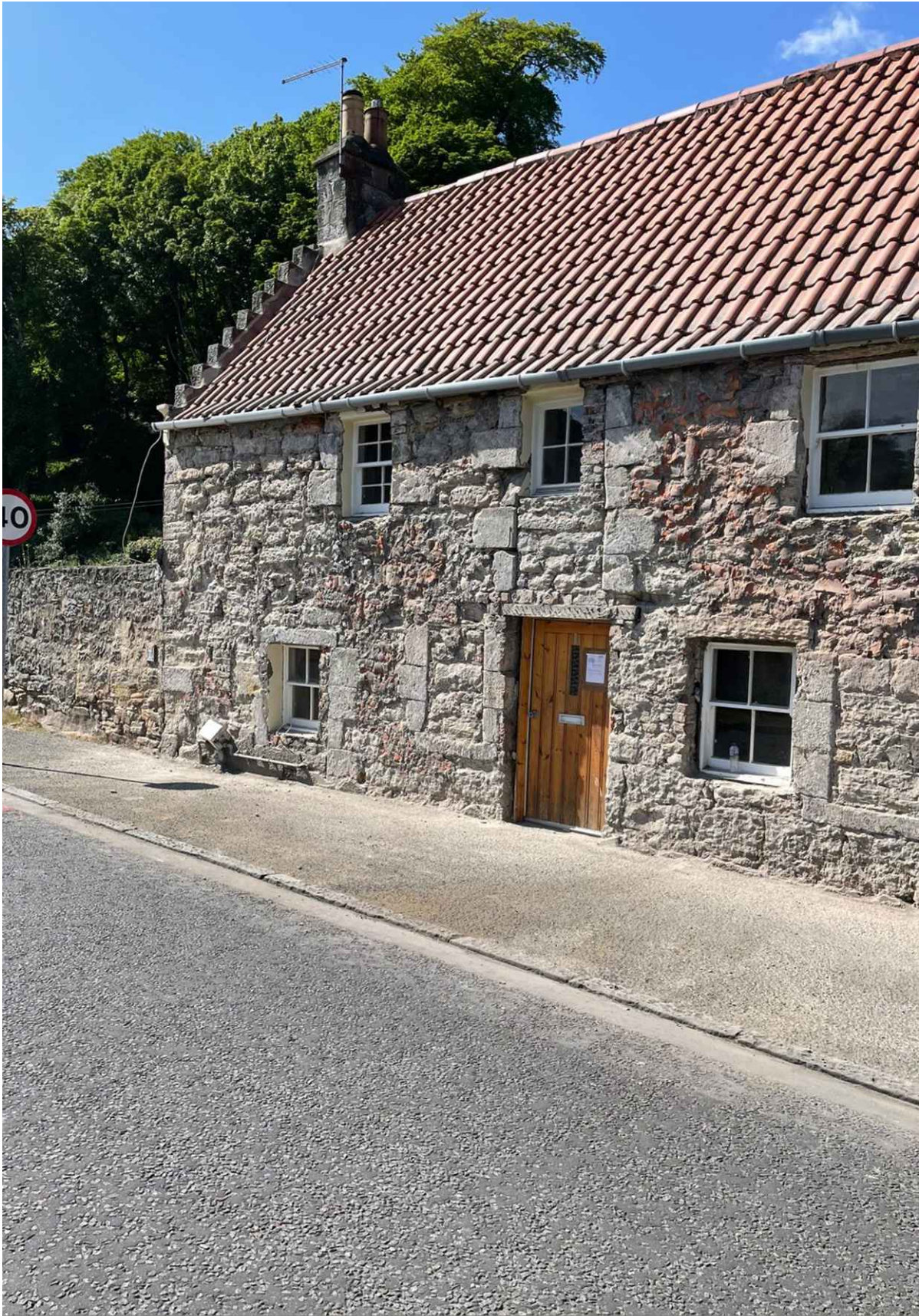
Original windows filled in with sandstone, either side of the front door. Quoins above the entry showing the infilled pend that once separated the two buildings. Brick and cement infill to fill in gaps in the wall for the cement render applied in the 1960's.
