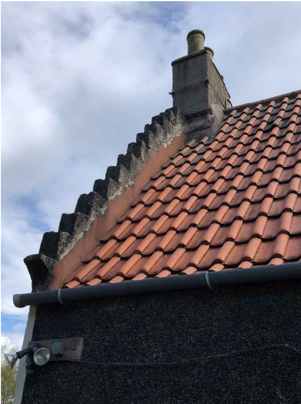
Change in roof line and pitch shown on north side at the east gable with cement flaring at the crowstep gable to make up the difference in the new roof line. This photo clearly shows the negative impact of the roof change in the 1980's without LBC and allowed water ingress into the roof space.
