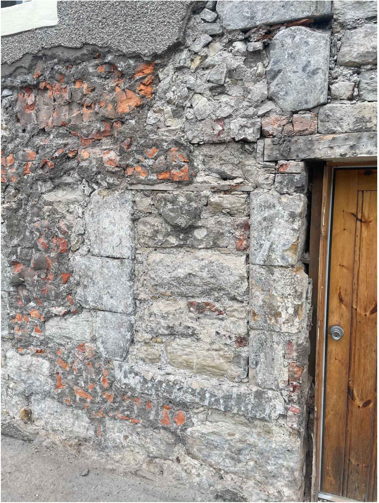
Original window filled in with sandstone to the west of the front door. Brick and cement infill to fill in gaps in the wall for the cement render applied in the 1960's.
