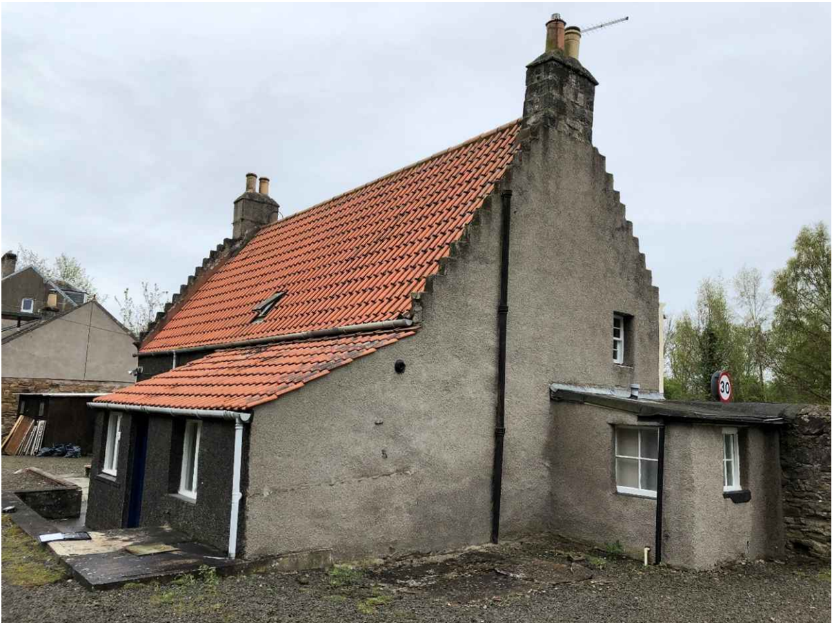
Figure 2: northwest corner of Westend Cottage showing kitchen extension to the north and bathroom extension to the west. The bathroom was constructed post listing without LBC.
