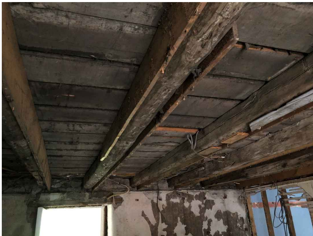
Sistered floor joists using 1" material. The floor joists were full of dry rot and had no load bearing capacity left. They had been sistered by timbers inadequate for their structural use and the resultant impact was a failure in structural integrity.
