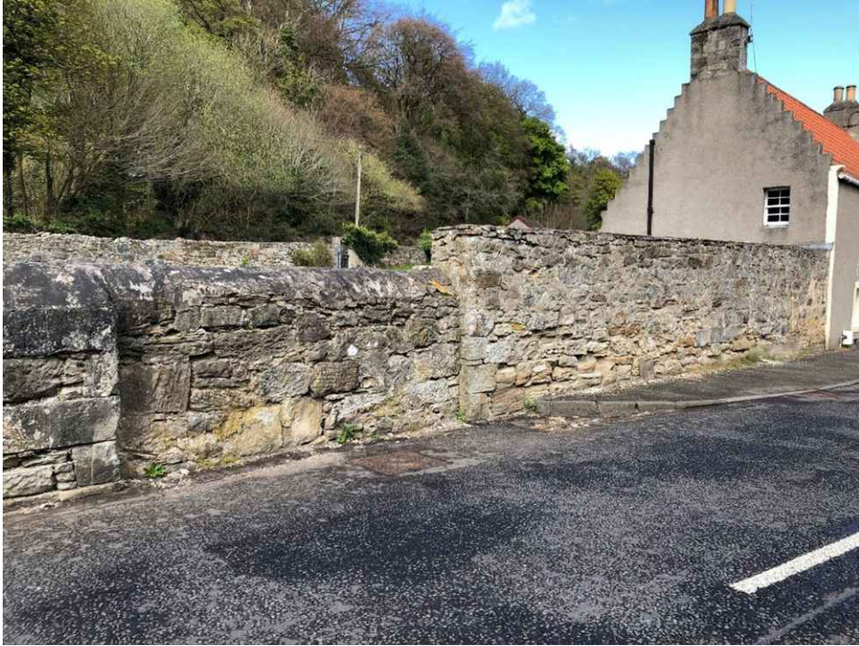
Figure 3: Part of south boundary wall showing original entrance to the property. The main south boundary wall is of the same depth and length as the existing cottage which could relate to its use as a former building at one time.
