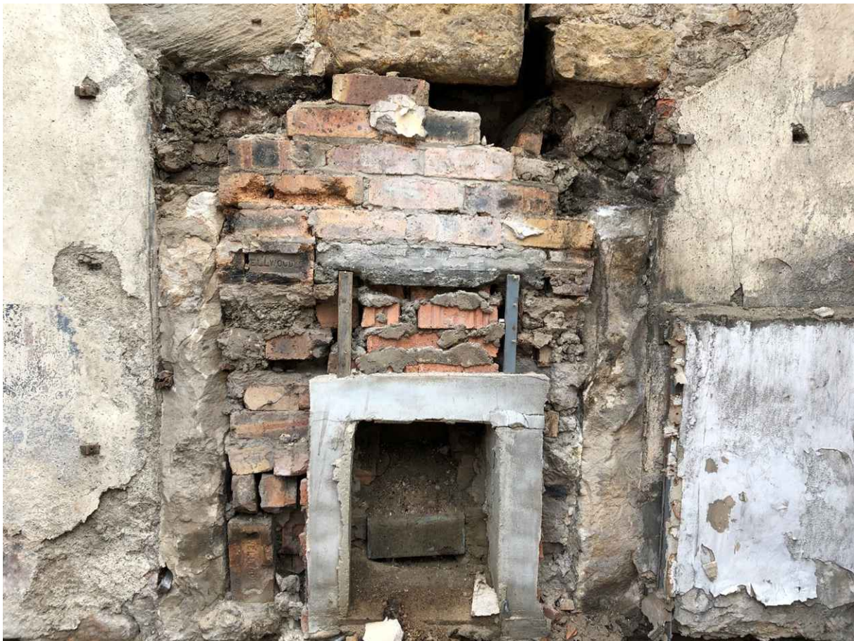
Original fireplace on the west gable exposed. The two stone columns are clearly visible, however, the stone lintel is missing. The stone lintel was replaced, and this fireplace will be retained and be a feature of the renovated property.
