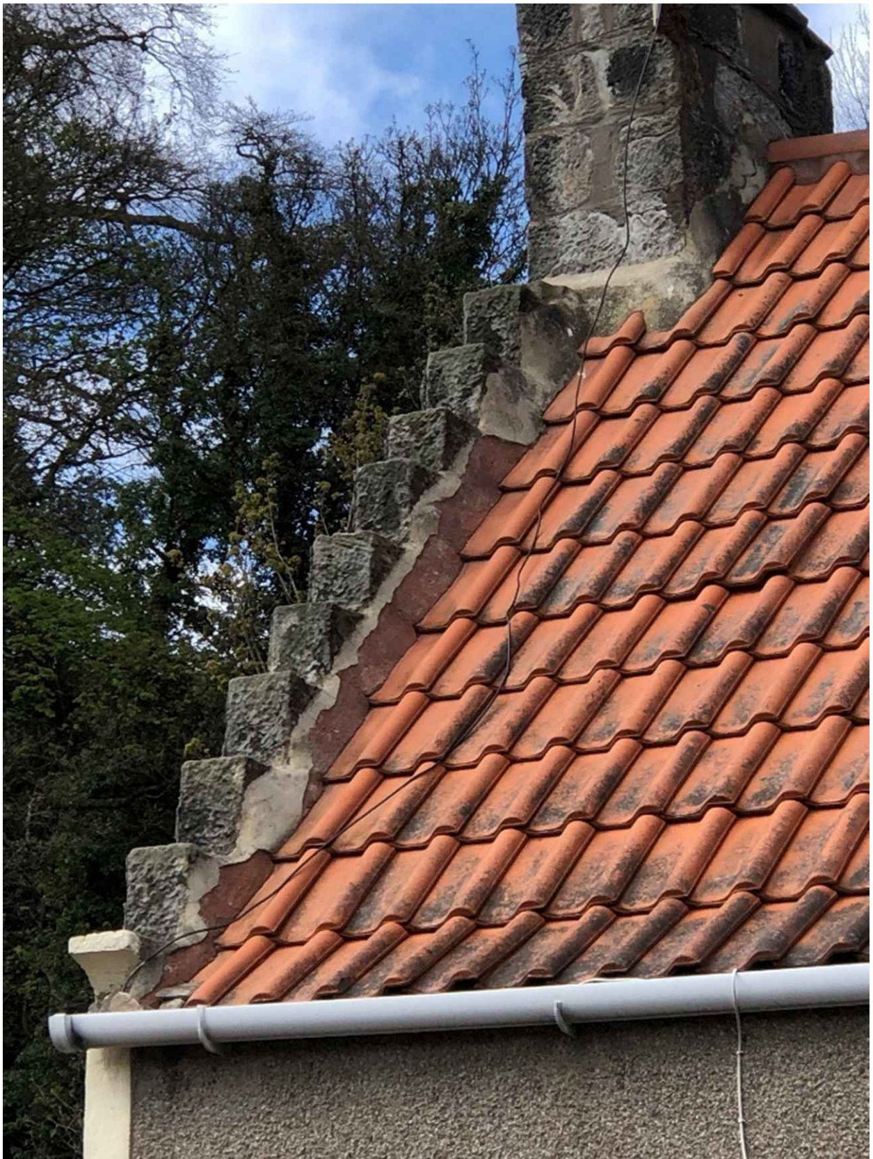
Change in roof line and pitch shown on south side at the west gable. The change of roof from the 1980's and poor workmanship at the crowstepped gable is clear.
