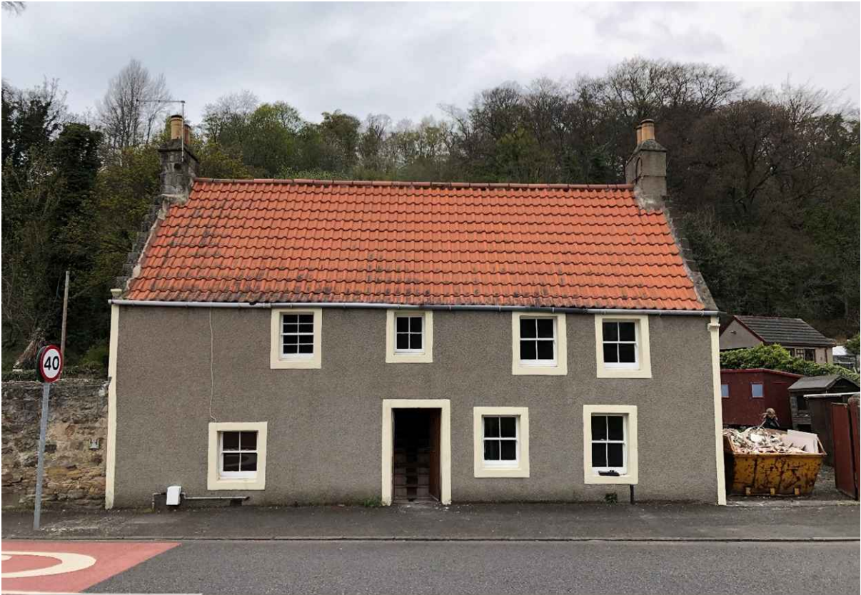
Figure 1: Westend Cottage, June 2023. Note the difference in pavement height and the resultant impact on the front door and front windows.
