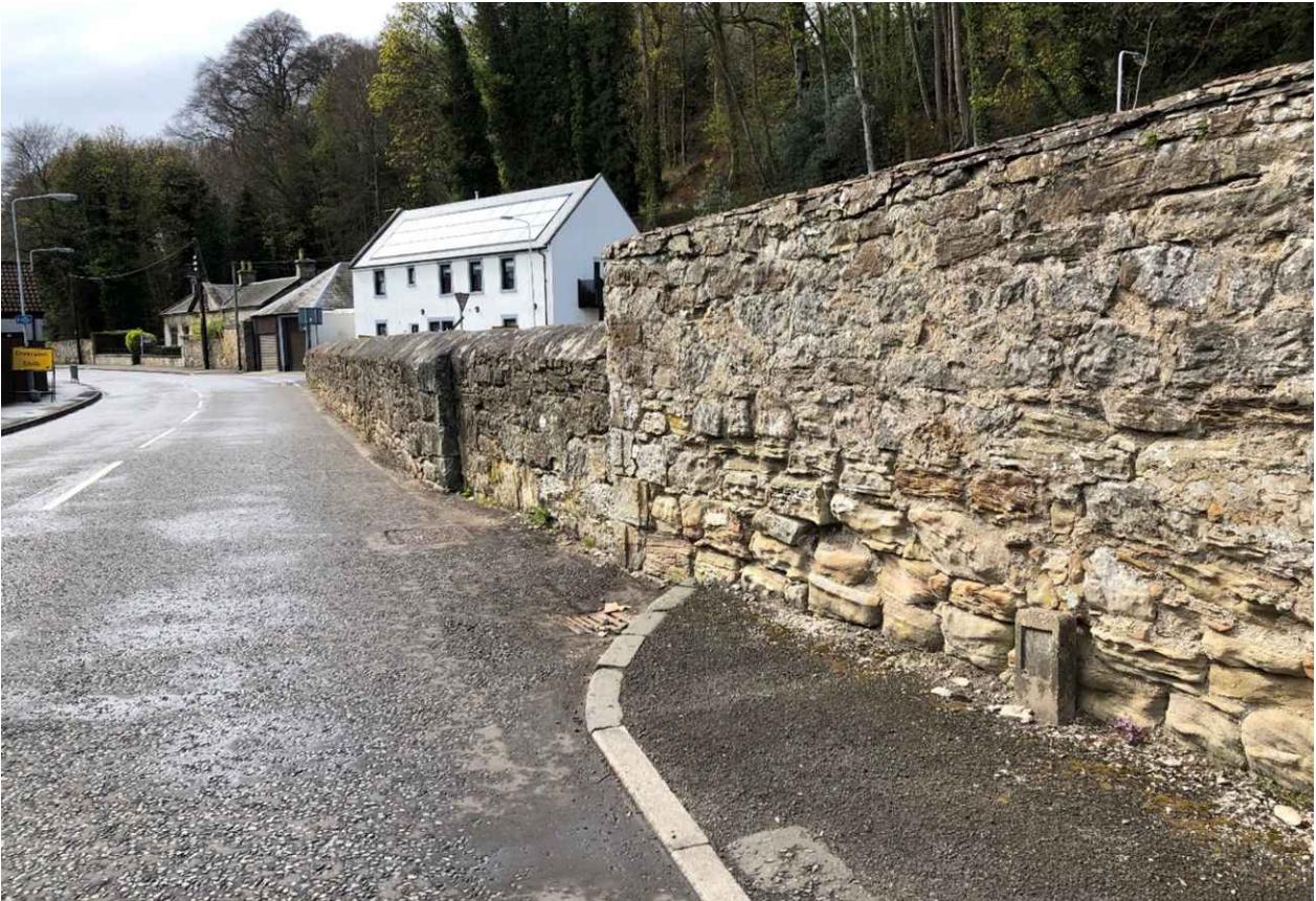
Figure 5: View west along Main Street towards Culross Conservation Area which starts beyond the curve in the road. Note: Saorsa Inn at the end of the property, which is full two storey and has no contextual relationship with Westend Cottage.
