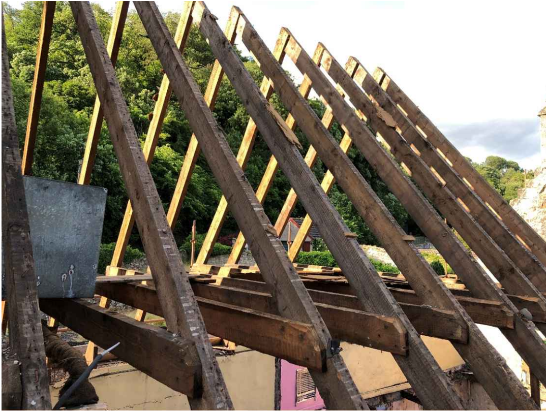
Exposed rafters after 1980's pantiles and substructure were removed post roof collapse. This was conducted outside LBC but was necessitated by health and safety concerns and the structural integrity of the exterior walls.
