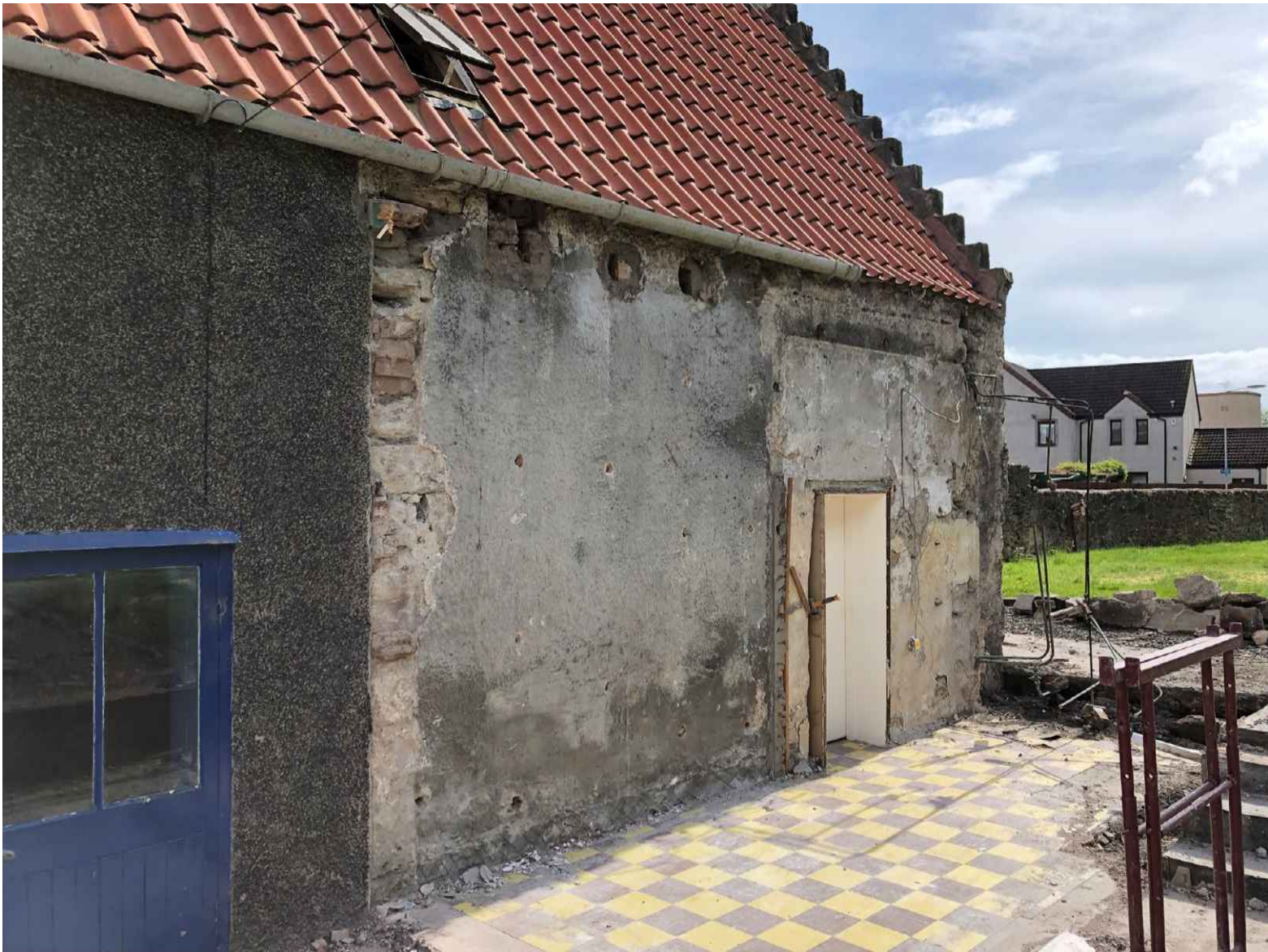
Figure 19:Rear wall of the original cottage once late Victorian kitchen has been removed. The image shows there was no keying in of the kitchen to the original structure
