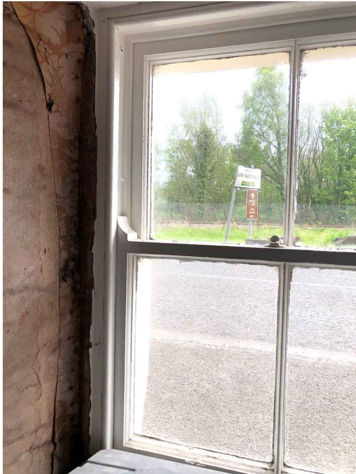
Figure 21: Image of window with stripped out box for sash and case so that the window fitted the opening. These windows were installed in the mid 20th century and are non-operational. Removal of the render as shown later dates window installation
