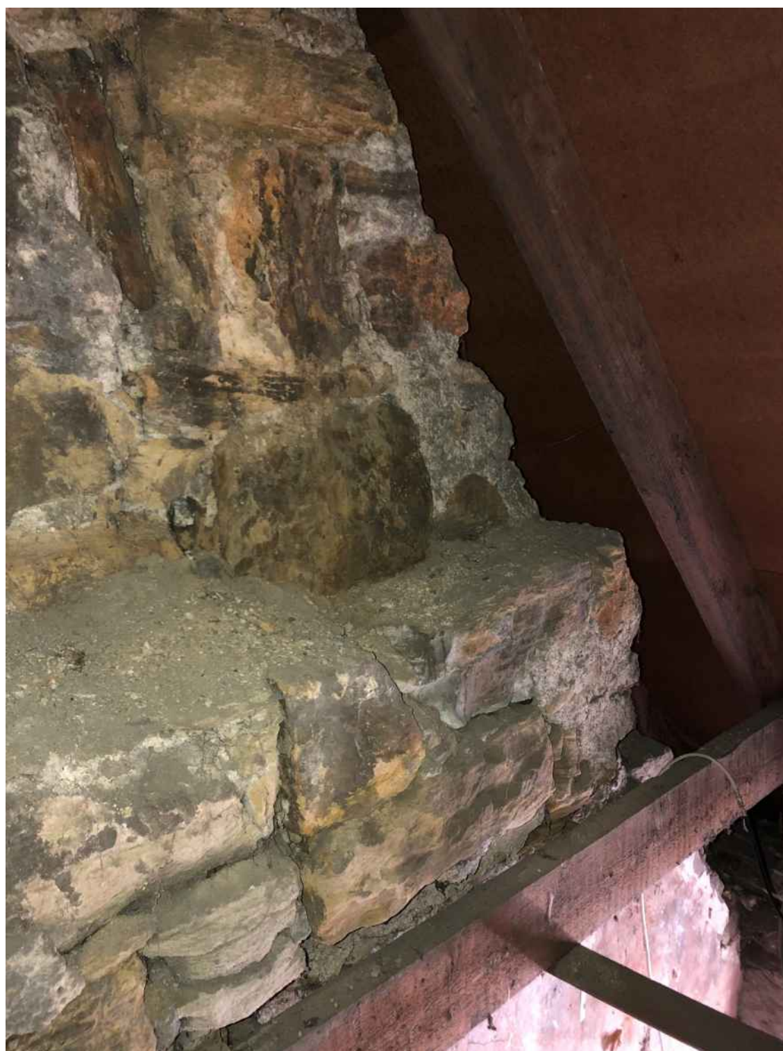
Figure 14: View of northwest gable wall behind 1980's timber trusses that shows the removal of stone in the rake of the gable to ensure the new roof fitted. This has had a negative impact on the listed building
