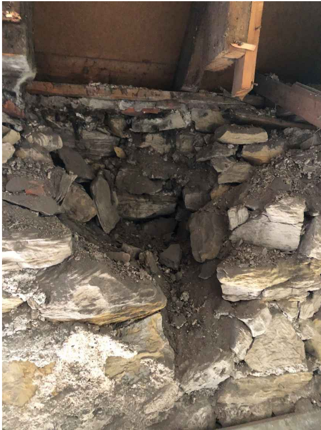
Figure 15: Loss of sandstone at the top of the southern wall head inflicted when the roof was installed in the 1980's and was covered by the subframe and t&g from the 1980's. Wall head to be repaired with local sandstone and lime mortar, NHL2.5
