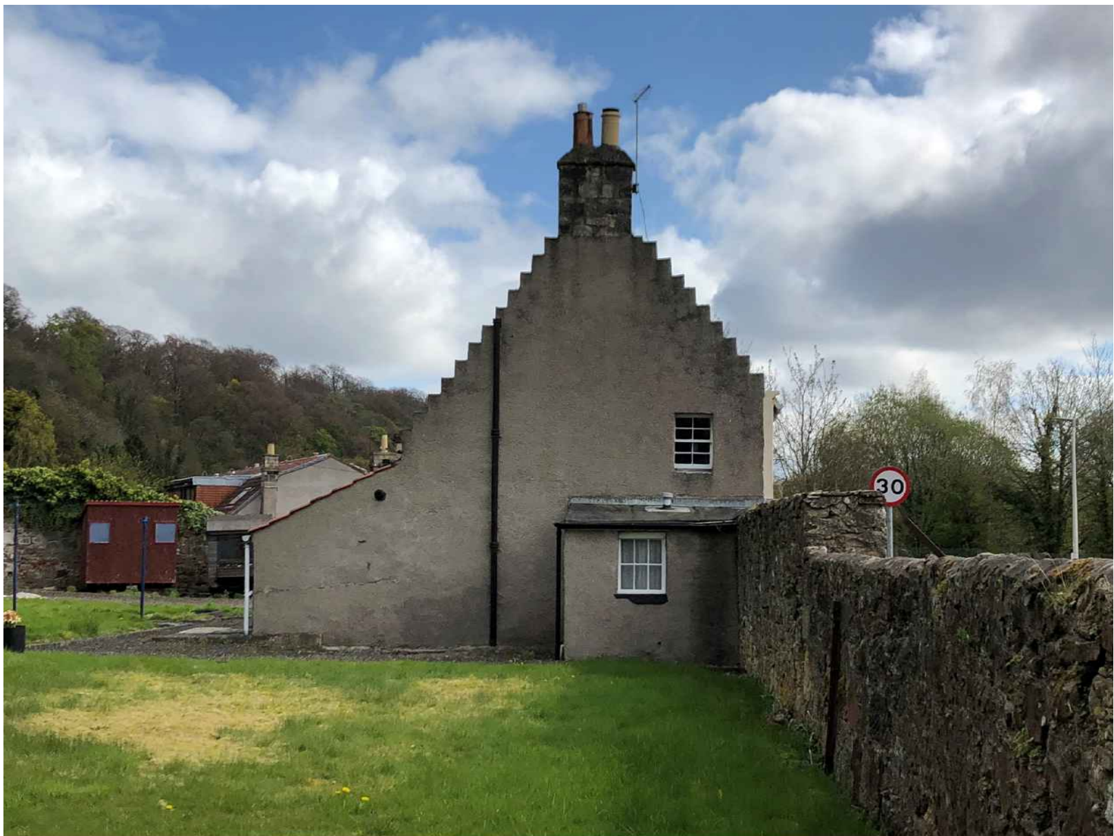
Figure 10: View of the west elevation of Westend Cottage showing the change in height of the southern boundary wall and the poor and leaking single storey bathroom extension built without LBC and against the boundary wall
