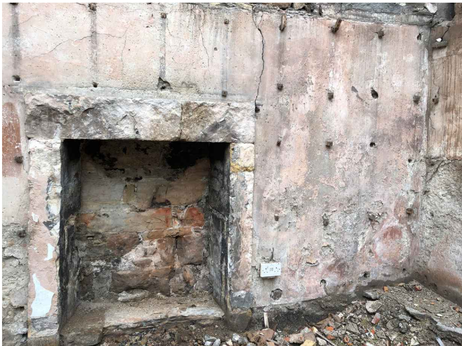
Figure 28: Image of uncovered original stone fireplace frame and lintel with stone grate and fire chamber on the east wall to be retained
