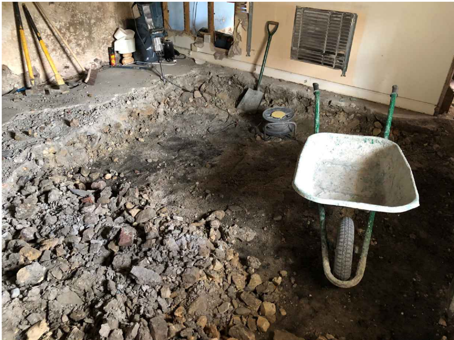
Figure 22: Excavation for the removal of the cement floor revealing the original grade surface with areas of fire charred remains. None of the original stone floor remained.
