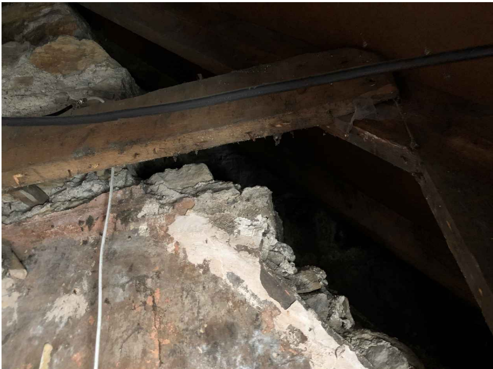
Figure 18: View of northwest gable wall behind 1980's timber trusses that shows the removal of stone in the rake of the gable to ensure the new roof fitted. This has had a negative impact on the listed building
