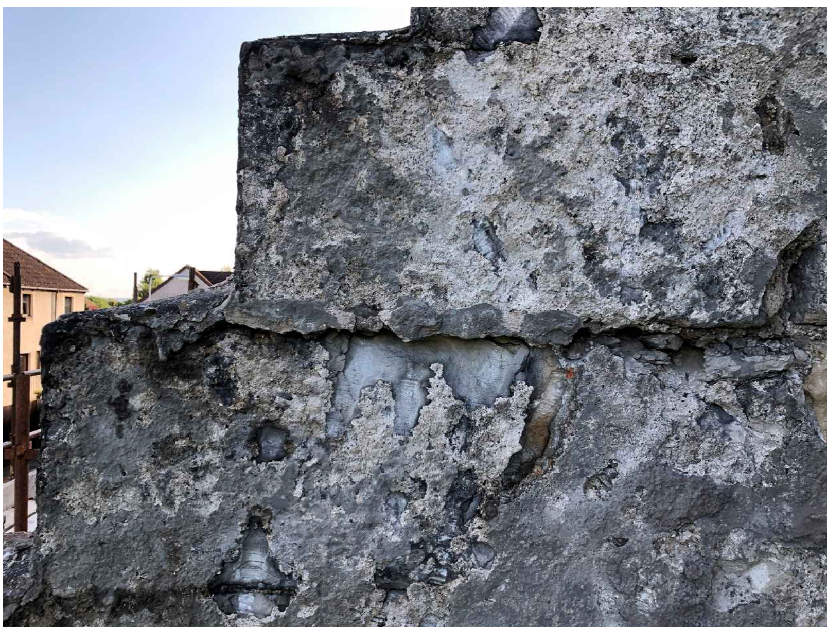
Figure 25: Crowstepped gables stone blocks hewn as individual elements of 500mm x 280mm each. Exterior Ashlar finish patina has been removed through poor workmanship when the roof and harling were installed
