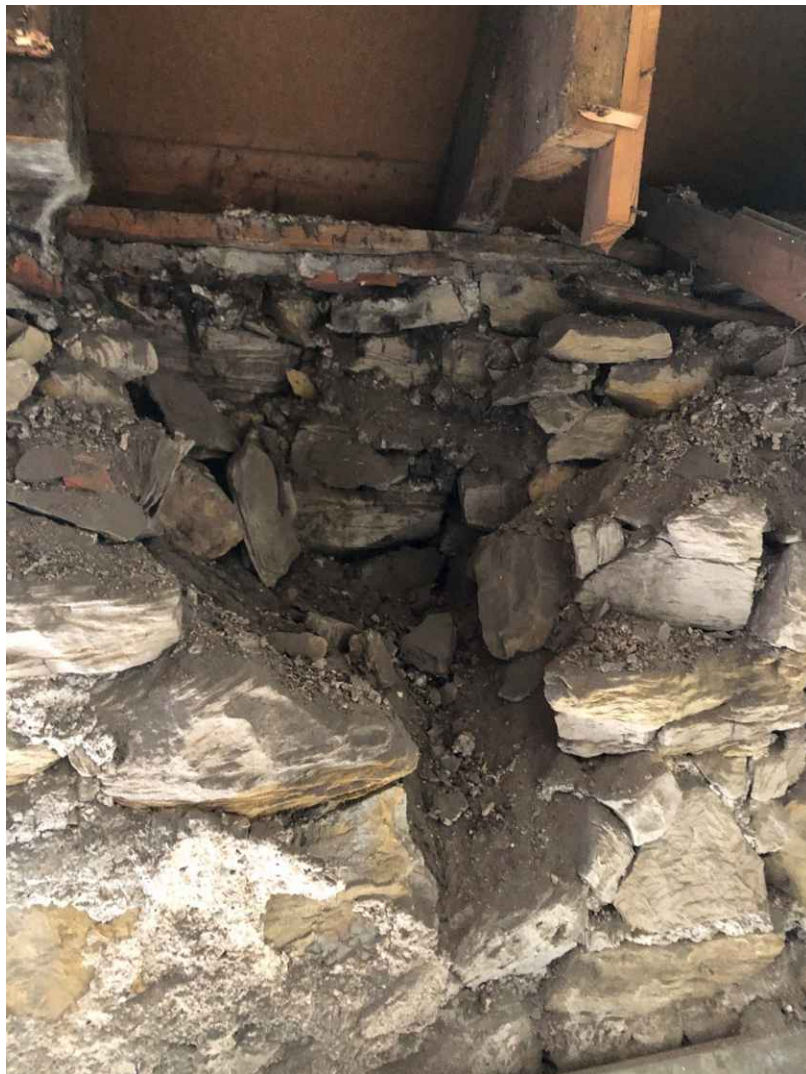
Huge hole in the first-floor south wall at the top of the wall head to the east of the front door. This area caused the roof to collapse during further renovation works. This was one of a number of voids discovered while work was ongoing.
