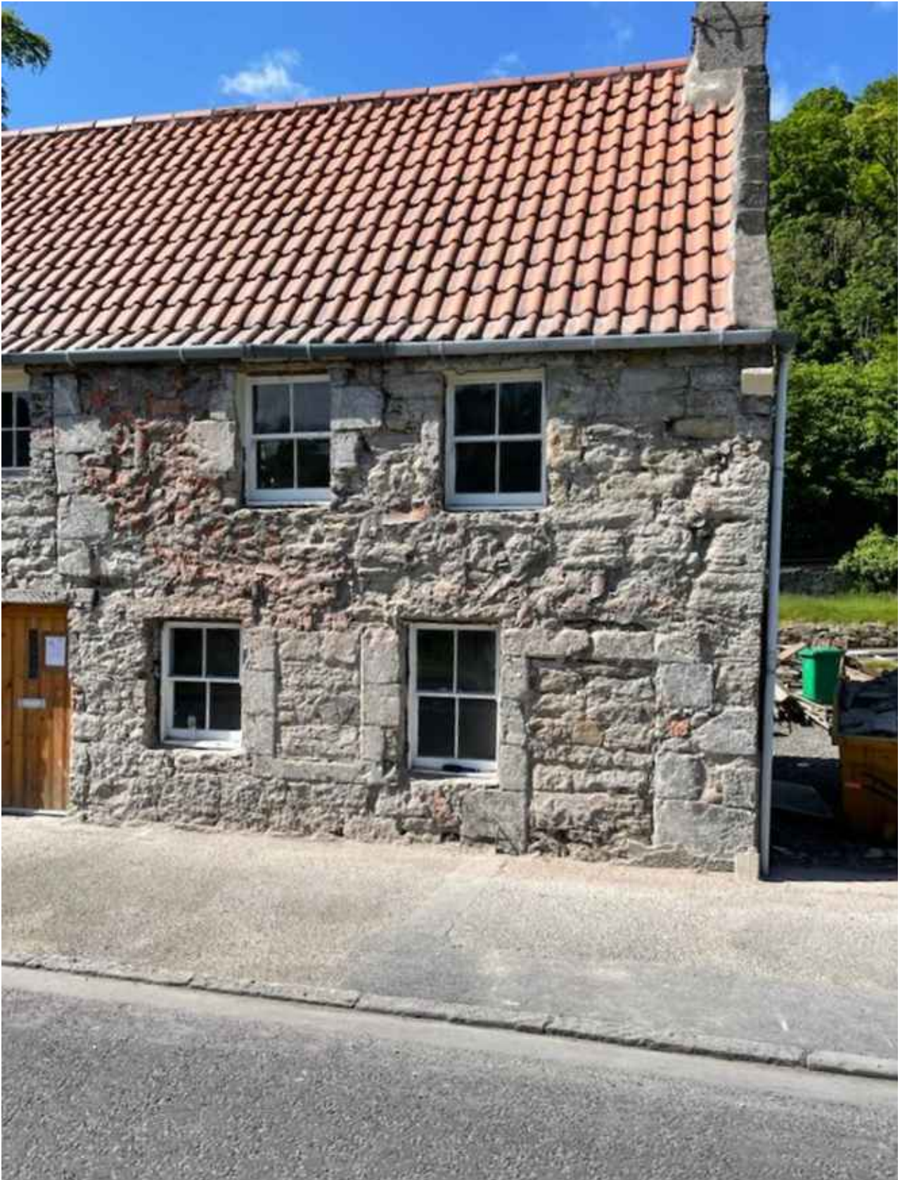
Original windows filled in with sandstone, either side of the front door. Quoins above the entry showing the infilled pend that once separated the two buildings. Brick and cement infill to fill in gaps in the wall for the cement render applied in the 1960's. The low skewput on the east side shows the change in the level of the wall for the new roof. There is also extensive damage to the sandstone from water and moisture impact.
