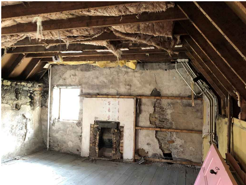
1 st Floor west bedroom. Stripping back to original wall construction. Note holes in the wall on the south side and at floor level from the exposed ground floor flue.
