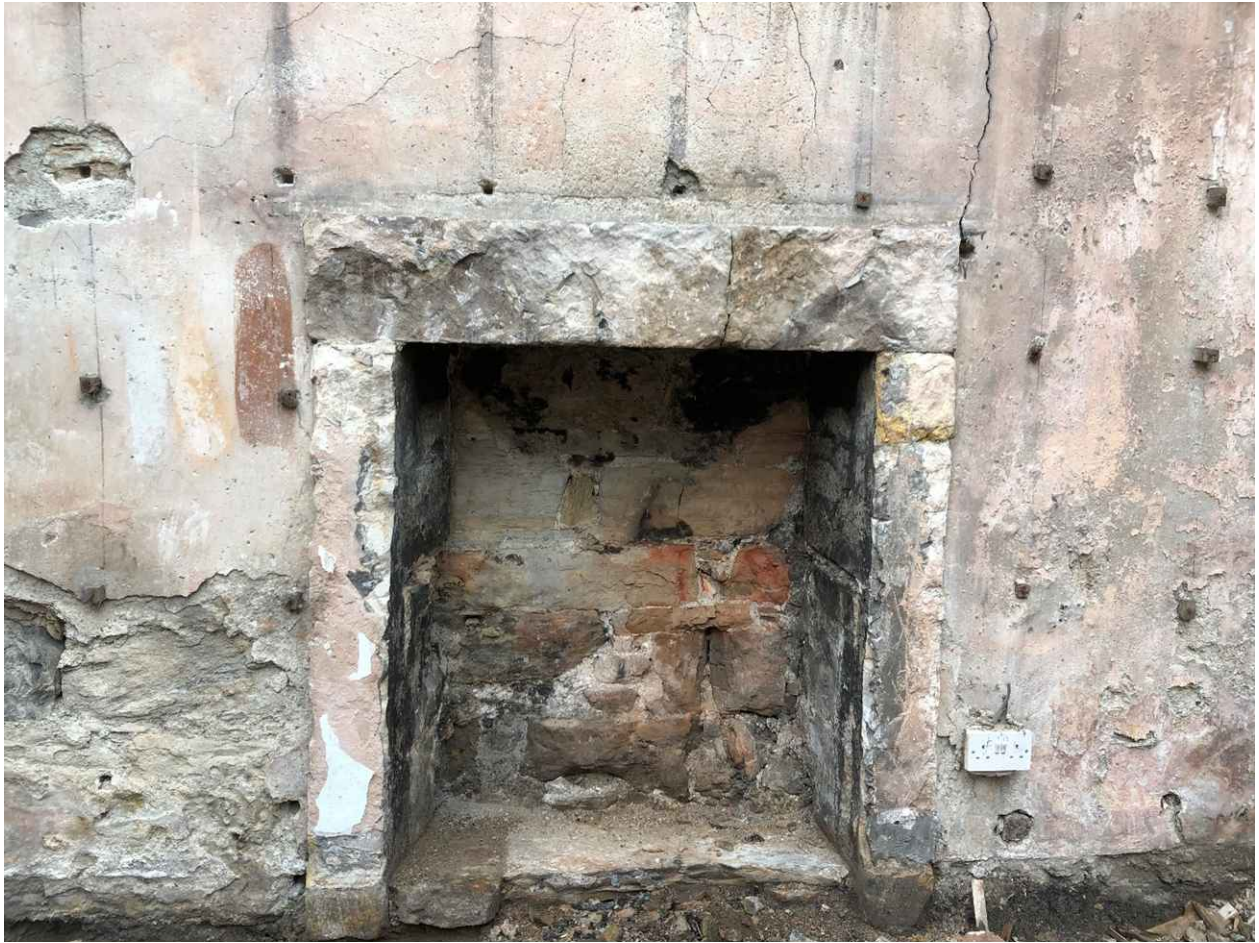
Original fireplace on the east gable exposed. Two stone columns and a stone lintel are clearly visible. These will be retained and be a feature of the renovated property.
