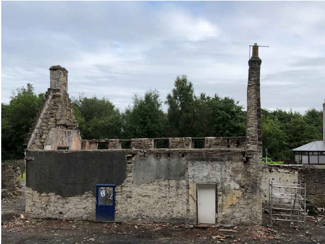
North elevation with roof removed. The west gable wall had shown signs of moving but this was deemed to be historical in nature. The wall head on the south wall has been repaired in three places with stone recovered from the site of the building. Both doors in this wall are not original to the house.
