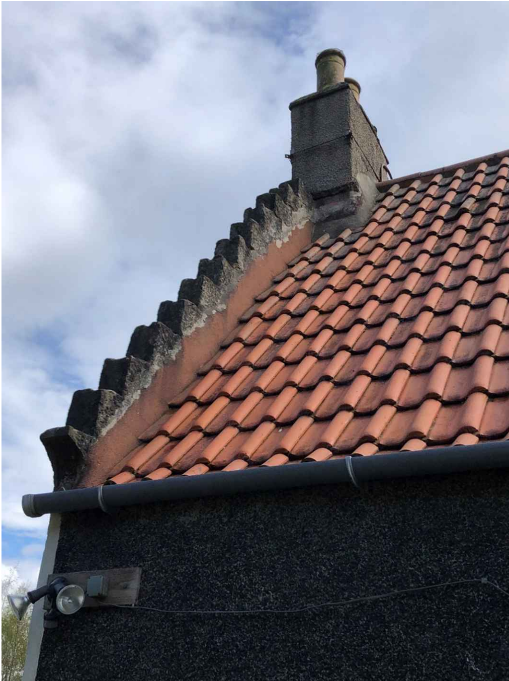
Change in roof line and pitch shown on north side at the east gable with cement flaring at the crowstep gable to make up the difference in the new roof line. This photo clearly shows the negative impact of the roof change in the 1980's without LBC and allowed water ingress into the roof space.
