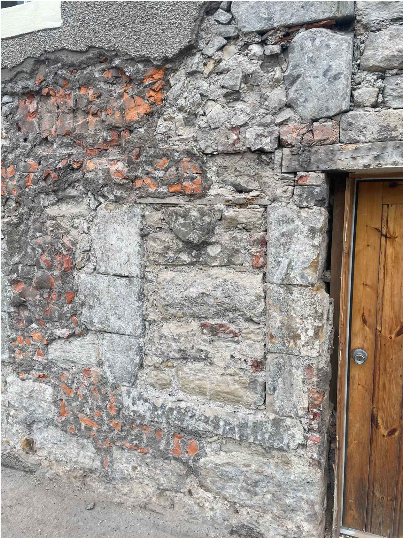
Figure 3: Original window filled in with sandstone to the west of the front door. Brick and cement infill to fill in gaps in the wall for the cement render applied in the 1960's
