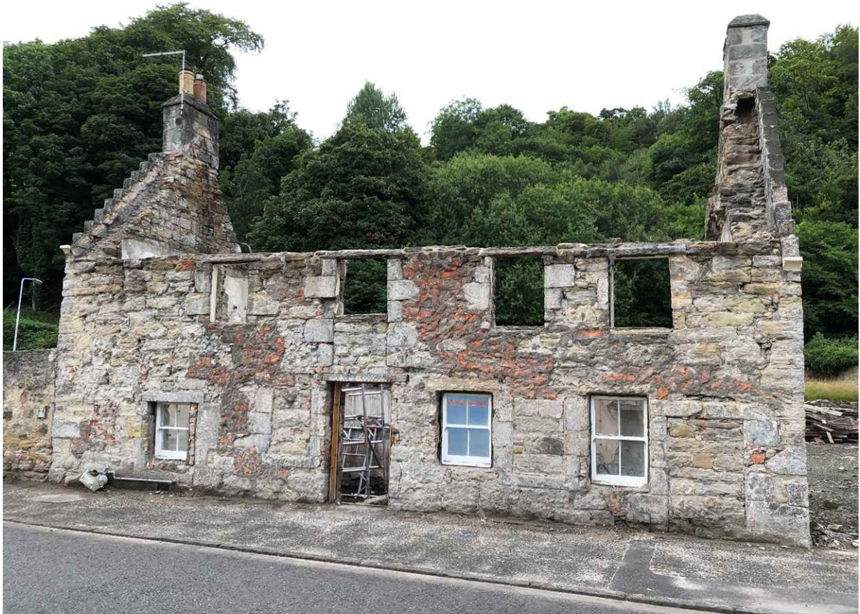
South elevation with roof removed. The west gable wall had shown signs of moving but this was deemed to be historical in nature.
