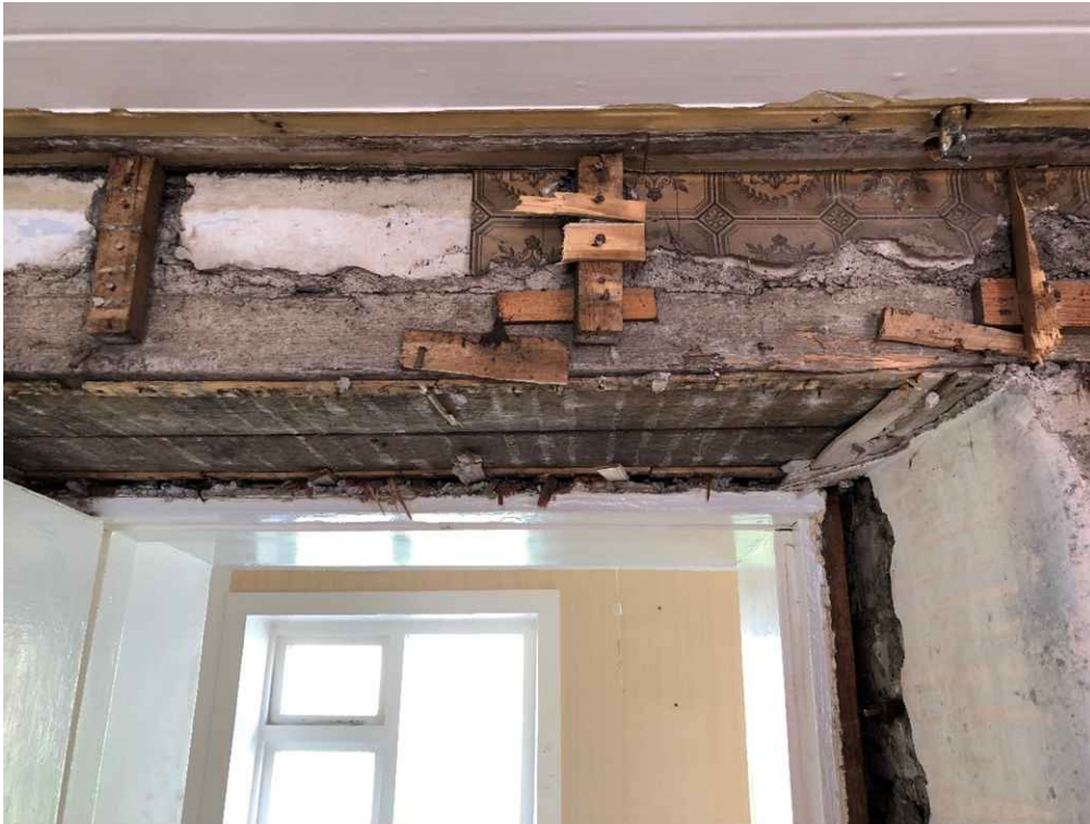
Doorway to kitchen showing timber lintel. This was not an original opening from the original cottage construction but was added in the Victorian period.
