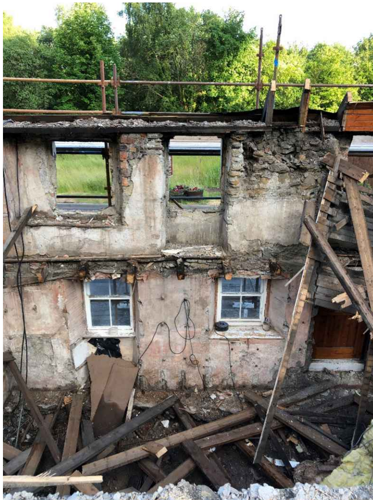
Image showing the top of the wall head that collapsed during interior works to the first-floor framing and exterior render removal. Pantiles had been removed at this point.
