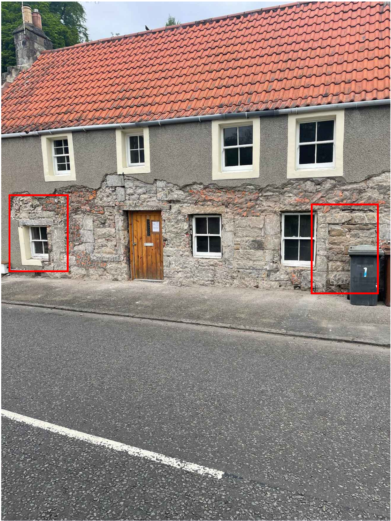
Lower render being removed from south elevation showing the original entrance on the east side and the original entrance shown on the west side of the south elevation
