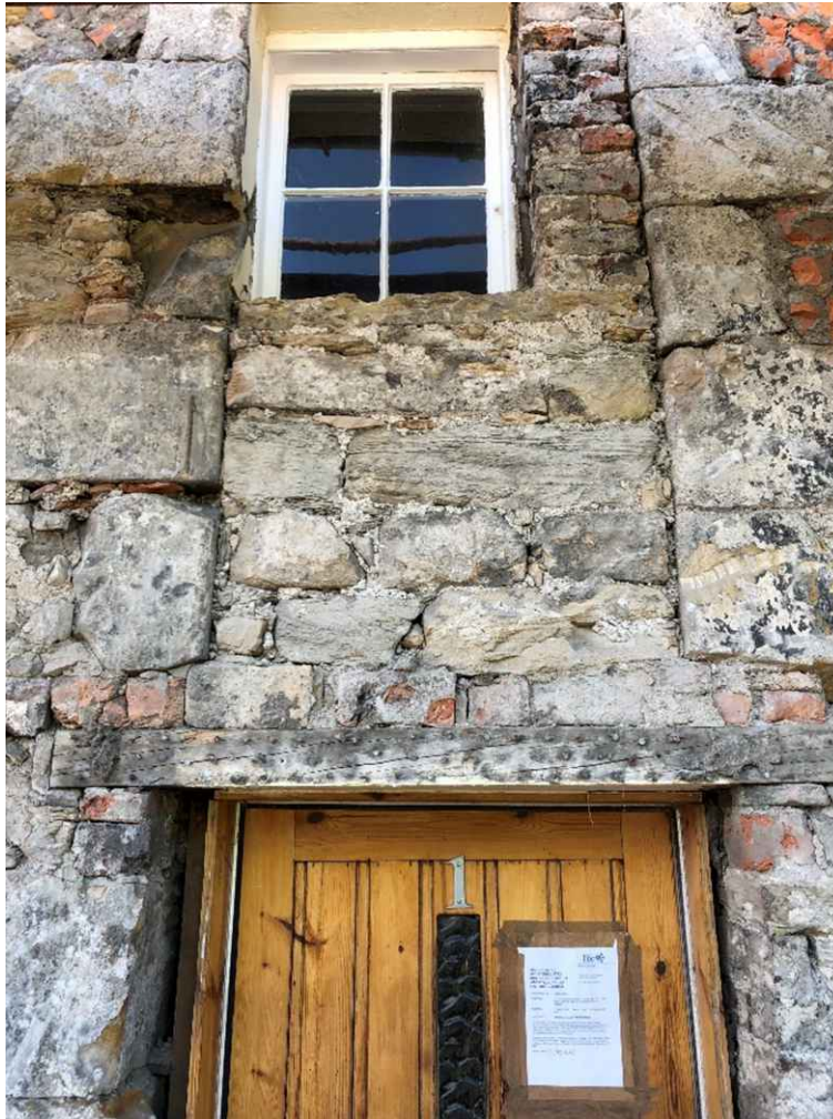
Quoined returns at the front door that show the building was once two distinct buildings. The quoins run down to grade
