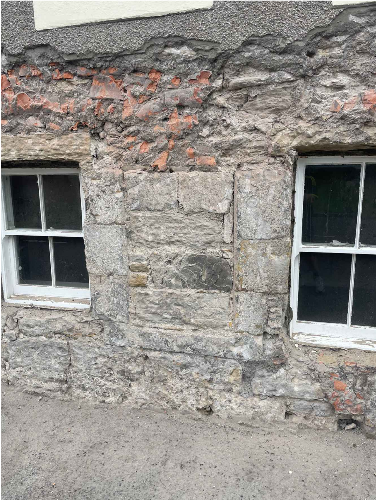
Original window on the west side of the south elevation filled in with sandstone. Brick and cement infill to fill in gaps in the wall for the cement render applied in the 1960's. The window opening adjacent to the original opening were added at a later date and the windows installed in the 1980's.
