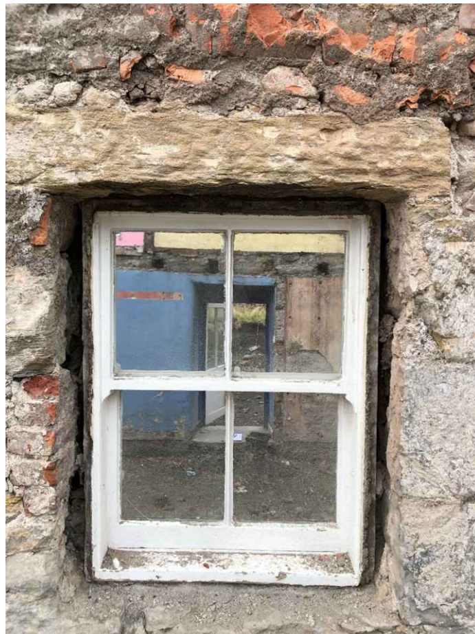
Once the render was removed from the wall, it is clear that the window was being held in place by the cement as the sash boxes were removed, therefore the window was sitting within the rough opening with no tieback. As the window was sealed closed and had no operating function, it served no function and is clearly not original to the building. This was deemed to be a health and safety concern as the window could easily fall out. These windows were retained in one of the rear sheds.
