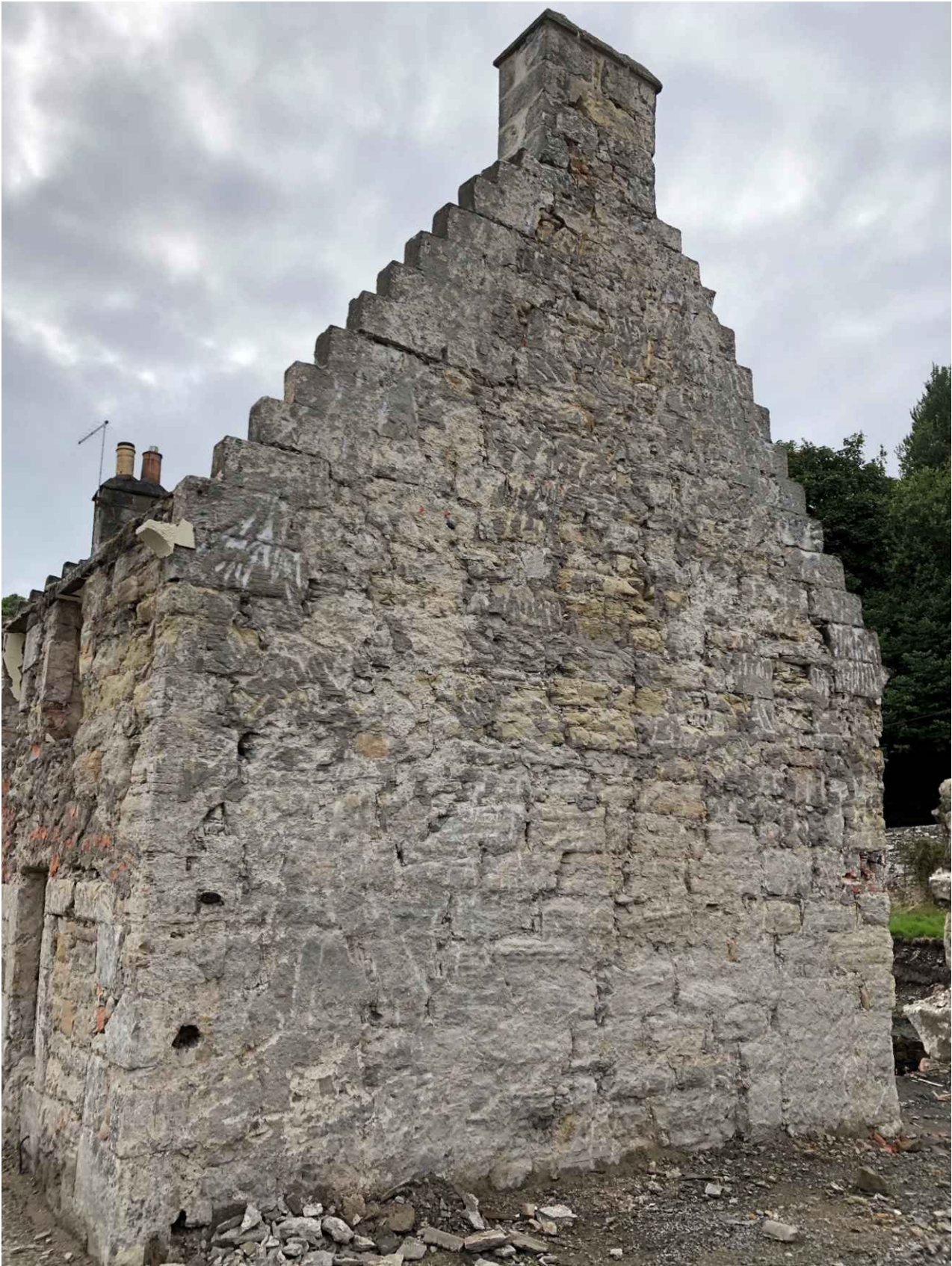
Figure 2: East gable showing original wall construction and skew puts at the same height indicating a typical symmetrical roof and building form. This gable also shows the impact of high moisture content within the walls.
