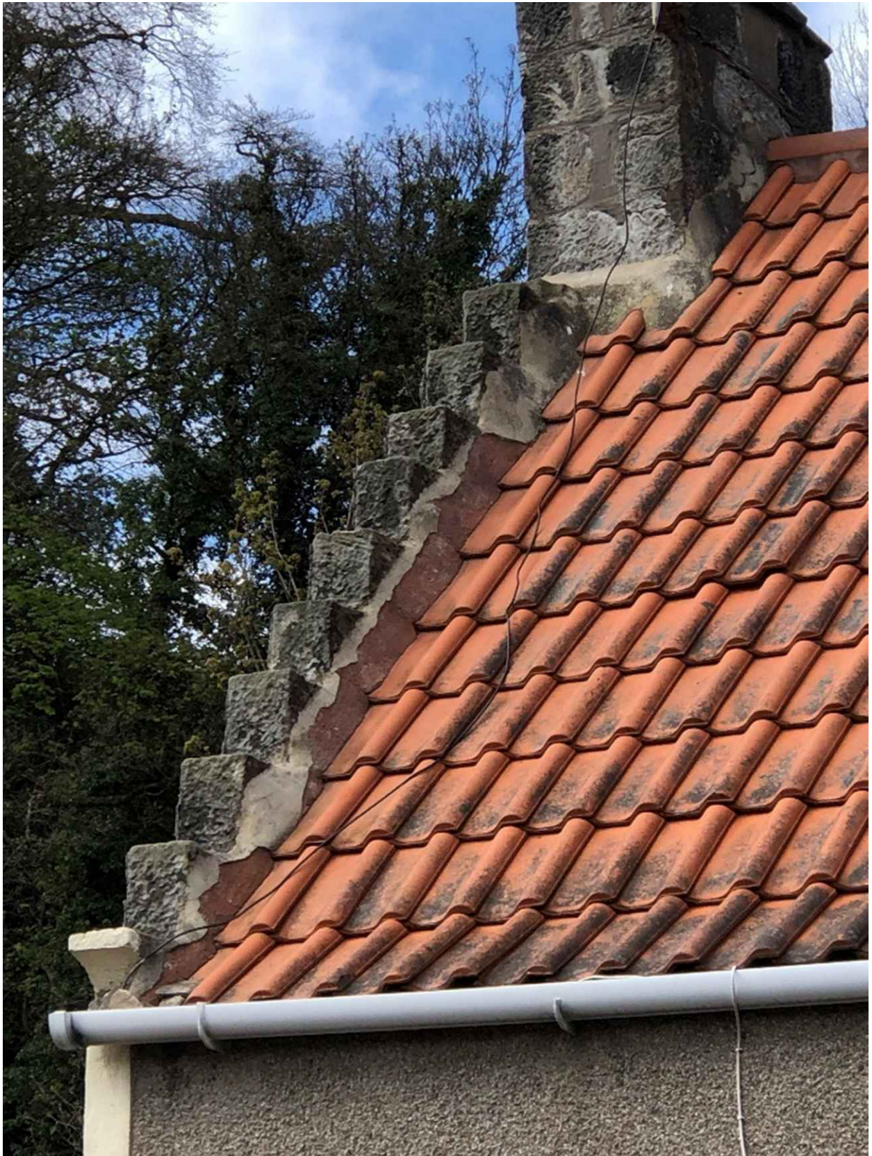
Change in roof line and pitch shown on south side at the west gable. The change of roof from the 1980's and poor workmanship at the crowstepped gable is clear.
