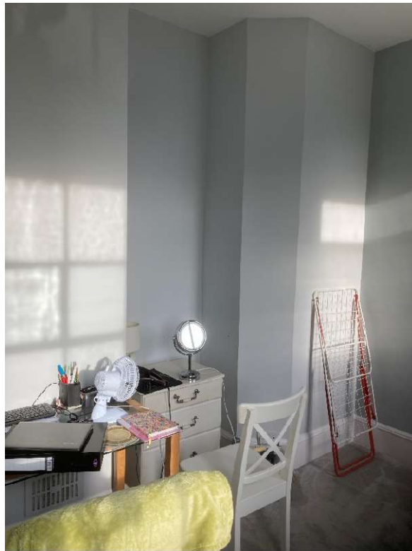
Fig.14 – Photograph taken in bedroom 2 showing the alcove where the original door was located
