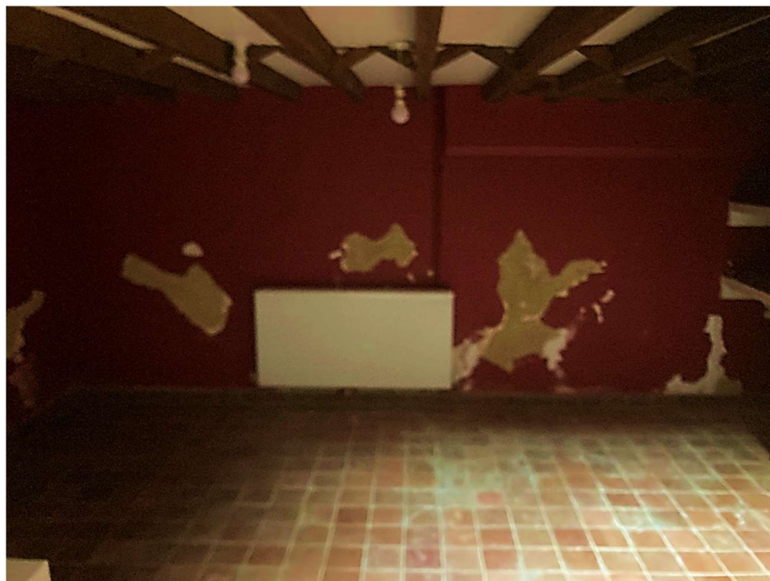
Fig.10 – Photograph taken in the basement showing the tiled and screeded floor and condition of walls
