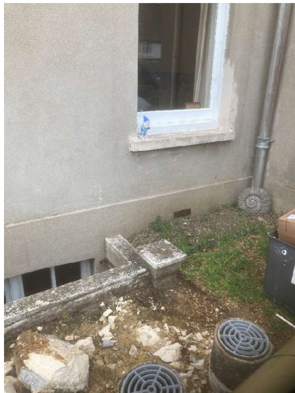
Fig.6 – Photograph showing the south-east elevation windows to the living room and basement (left)
