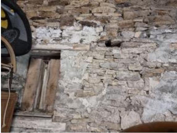
Figure 20: example of holes in walls.
