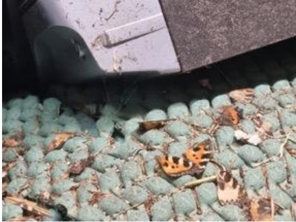
Figure 14: B1 - example of insect wings on stored items in building
