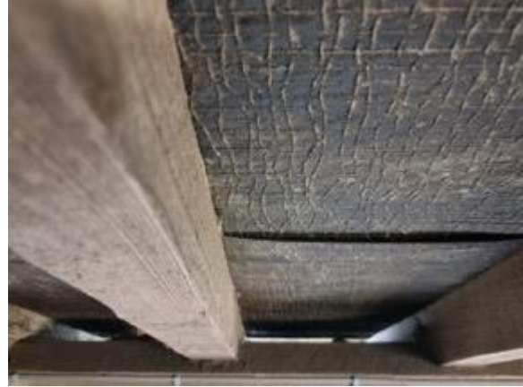
Figure 21: gaps under eaves
