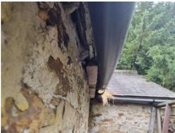
Figure 22: gaps under eaves from outside.
