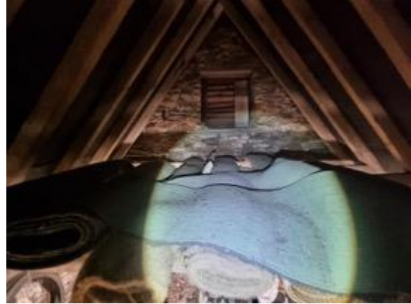
Figure 15: B1 - Bat droppings under roost (on stored carpets)
