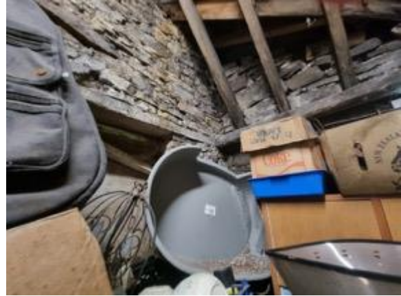
Figure 27: inside of front/E of building. Shows connection of coal shed to roof.
