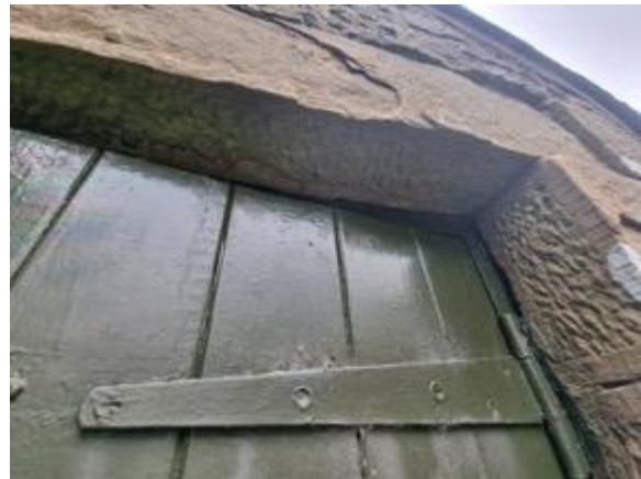
Figure 25: gaps around edges of doors
