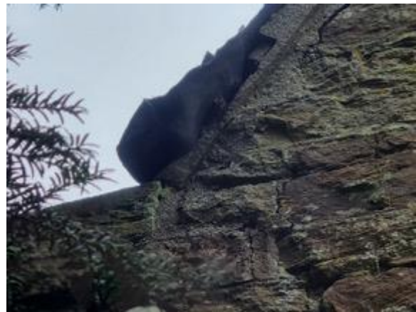
Figure 23: gaps at west edge of south gable end.
