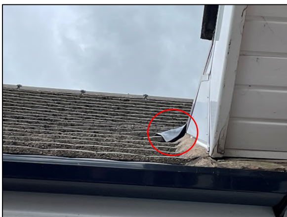
Plate 5: lifted lead flashing on B1 presenting Potential Roosting Feature (PRF) for bats.
