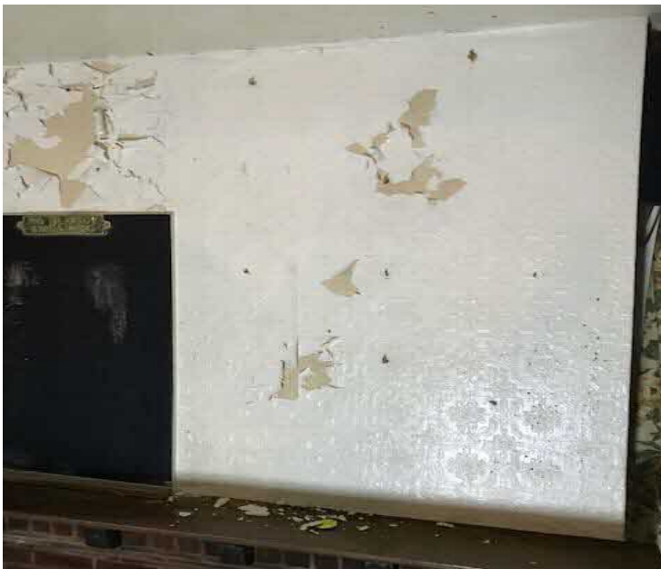
Sample 08 – Flaking paint - No asbestos detected.
