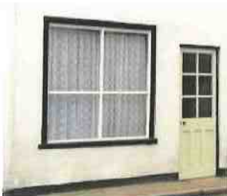
Original window before damage
