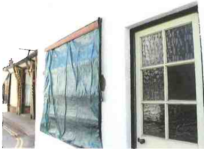
Damaged window boarded up
