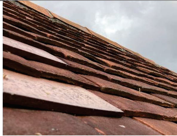
Photograph 2: Hand-made roof tiles on the eastern elevation as seen out of the pitched roof windows
