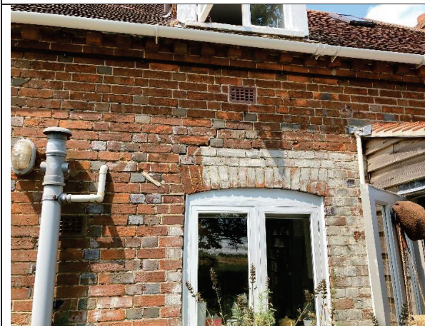
Photograph 3: Mortar gaps in the ground floor brickwork
