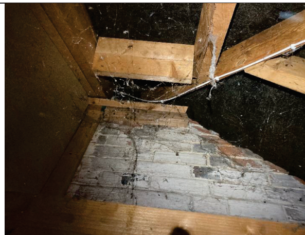
Photograph 4: The first roof void showing heavy cobwebbing
