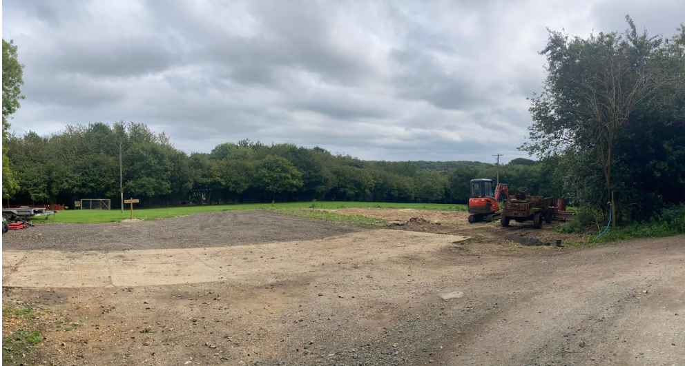
Image 4 – Cleared and tidied site. The former dwelling and approved replacement dwelling being situated where the orange digger is parked.
