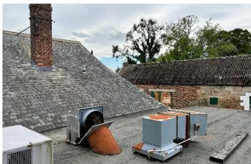
Previous array of ventilation units on roof
