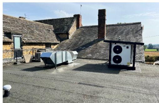
New array of ventilation units & ASHPs
