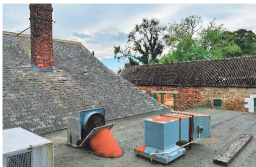
Previous array of ventilation units on roof
