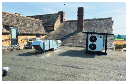
New array of ventilation units & ASHPs
