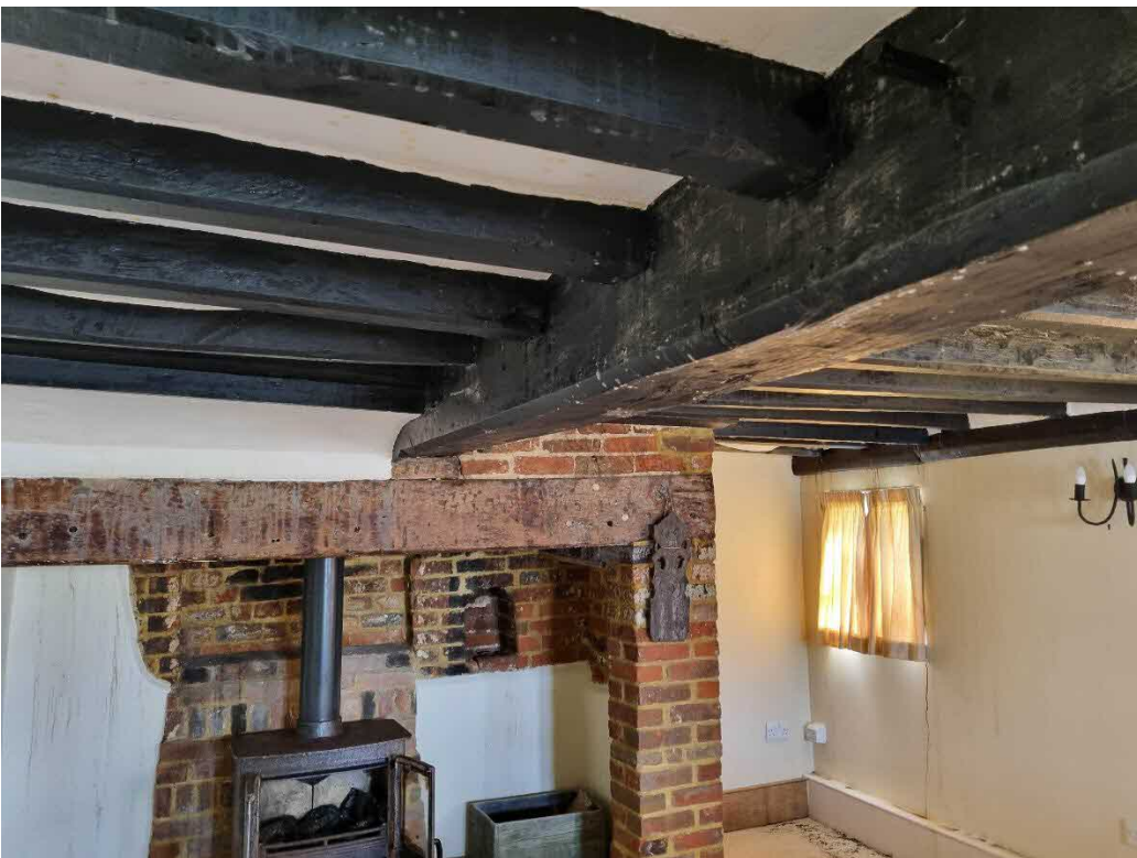
PHOTO 006 Internal view. Ground floor not affected by fire.
