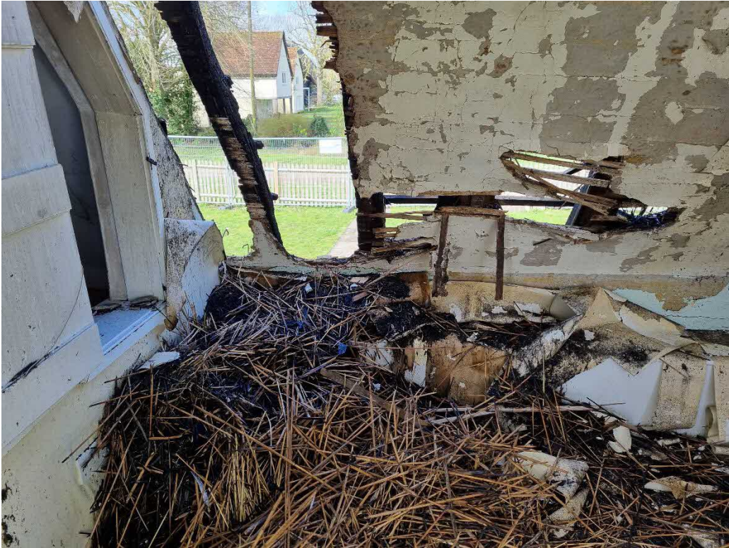
PHOTO 003 Internal view. Damage to roof.
