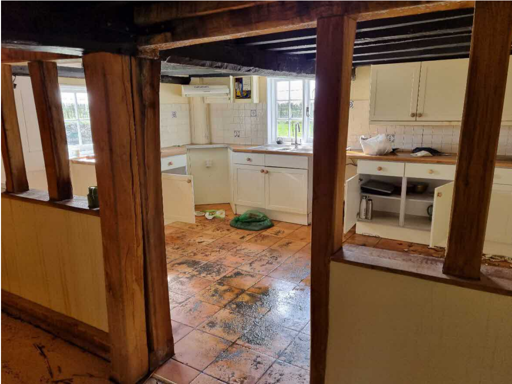
PHOTO 007 Internal view. Ground floor not affected by fire.
