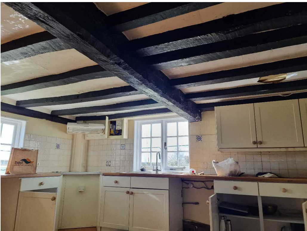
PHOTO 008 Internal view. Ground floor not affected by fire.
