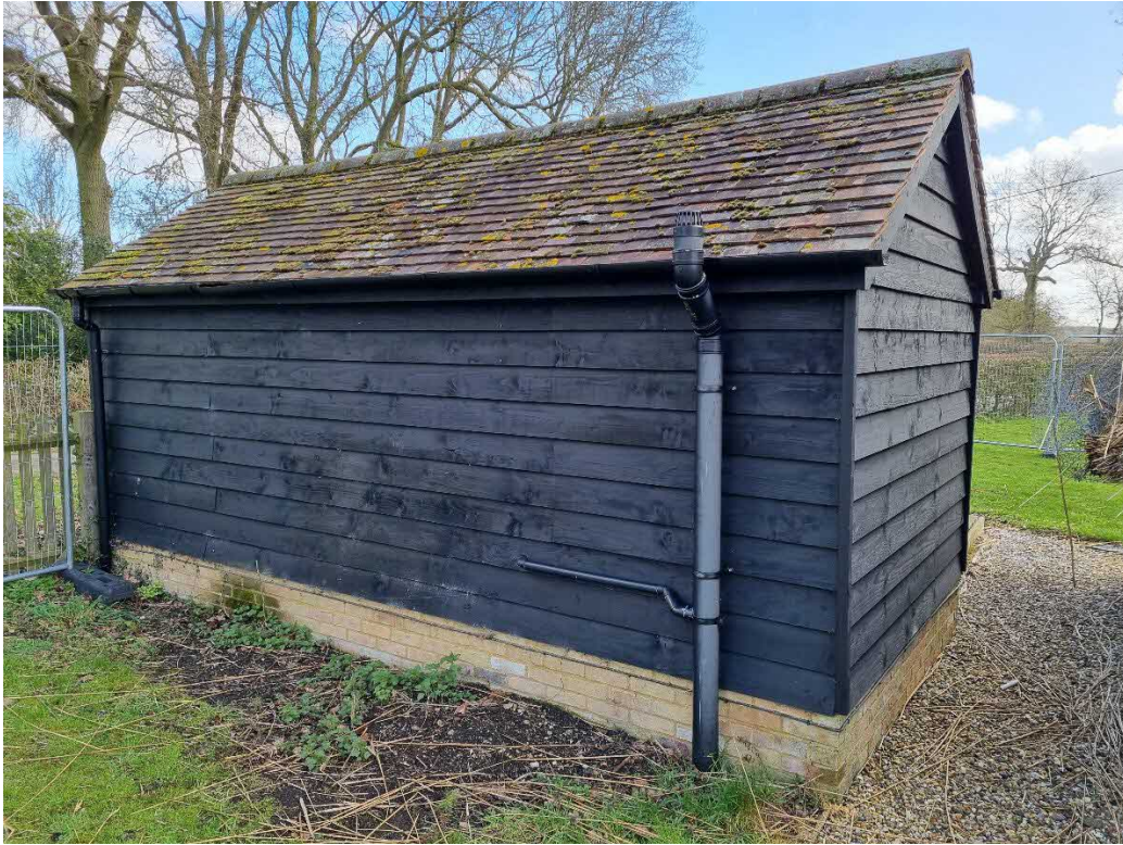
PHOTO 011 External view. Existing shed not affected by fire.
