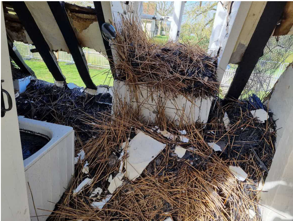
PHOTO 004 Internal view. Damage to roof.
