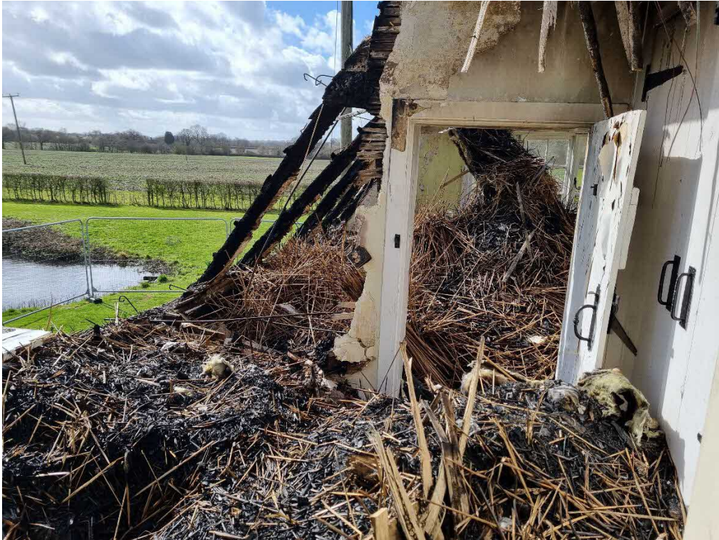
PHOTO 005 Internal view. Damage to roof
