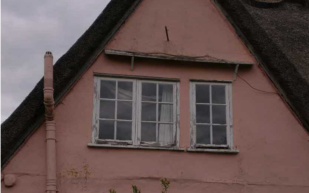
Fig. 1.2.3 showing first floor bathroom gable window with disintegrating bottom rails and inadequate decoration/maintenance - also note Upvc S&VP which is to be removed
