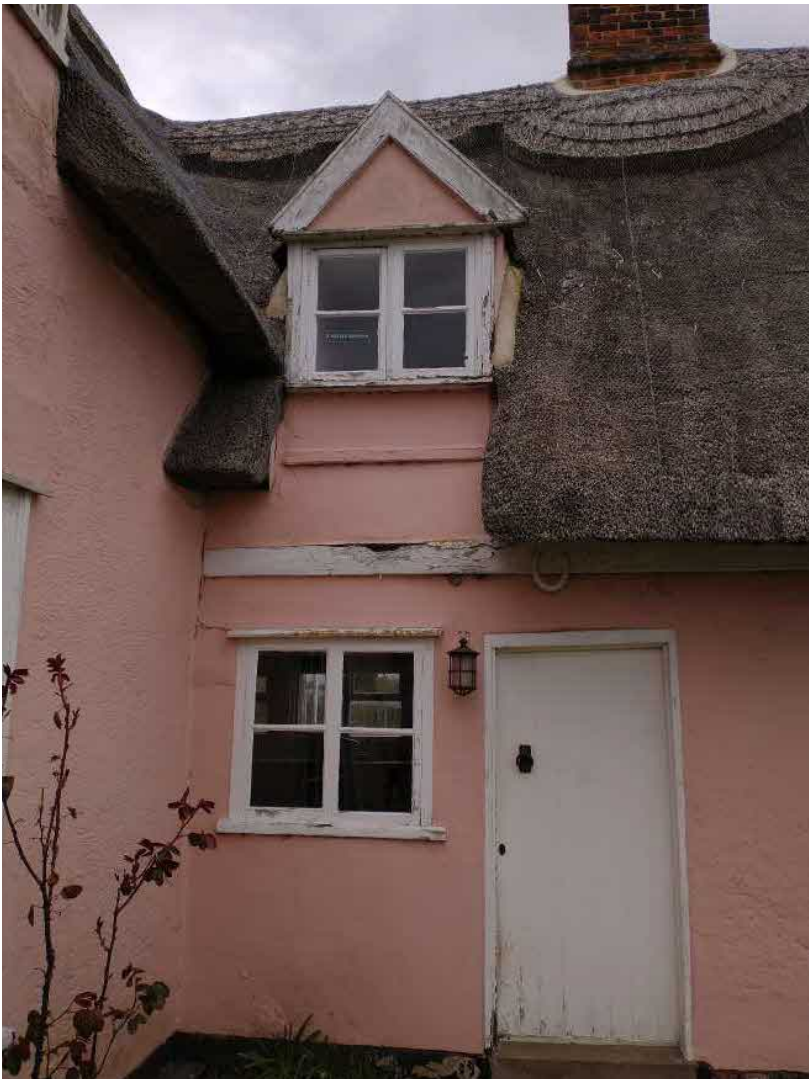
Fig. 1.2.4 showing large gap and rot in the horizontal timber above kitchen door, also note poor state of window and dormer joinery decorations
