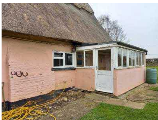
Fig. 2.2.1 Existing modern, felt floor at roofed 1970s utility room extension of no architectural interest and poor quality construction to be demolished to improve the west elevation
