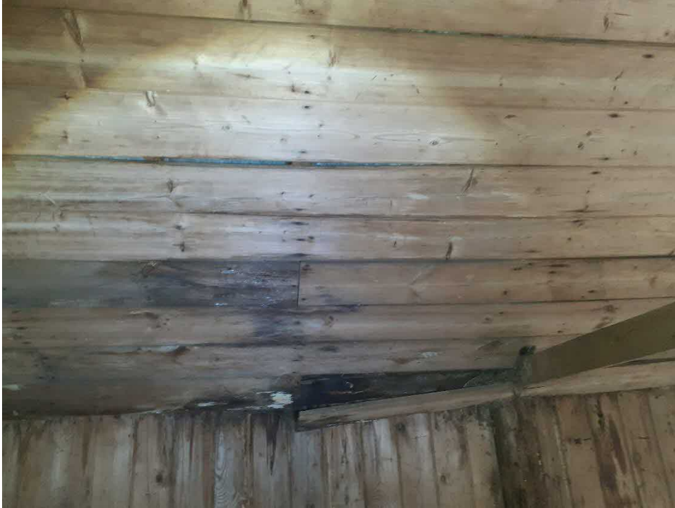
Photograph 39: Gap between the wooden ceiling panels of Building 2
