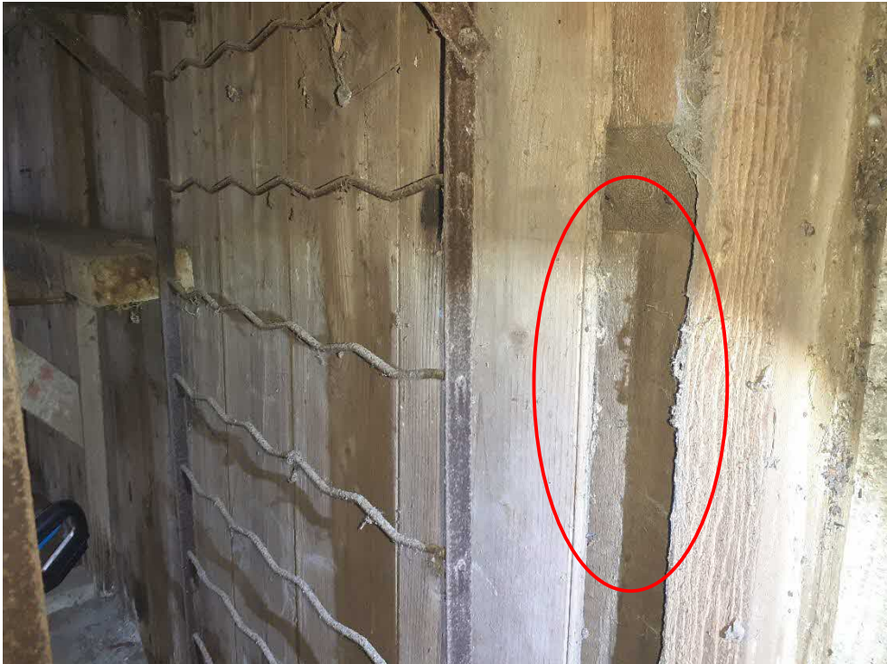
Photograph 36: A view of the cavity, and potential roosting feature, which exists between the interior and exterior wooden panelling of Building 2
