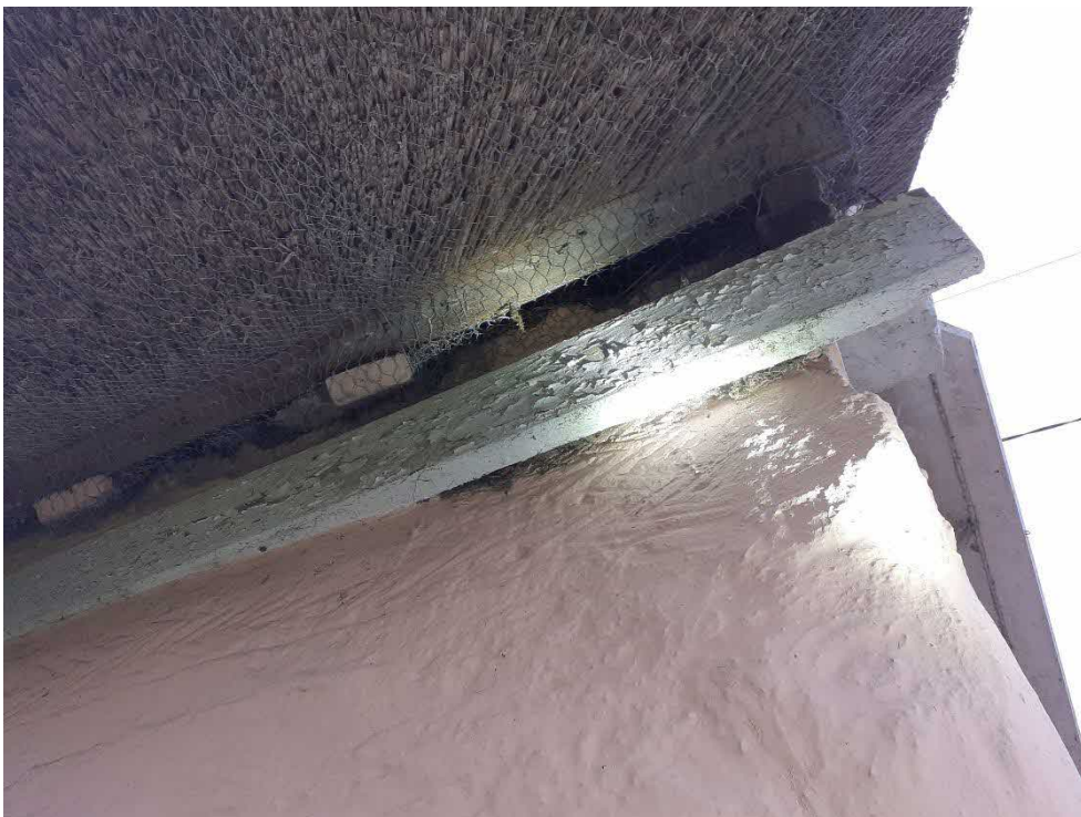
Photograph 21: An area under the eaves of Building 1 which has been sealed with chicken wire
