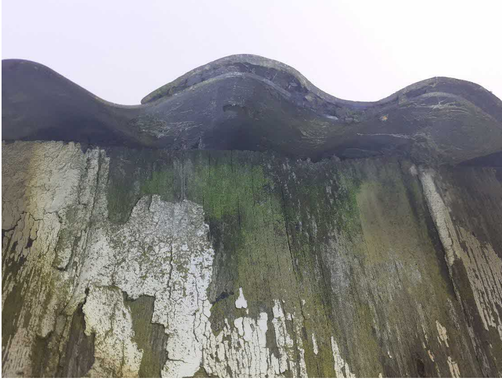
Photograph 35: Metal gaps beneath corrugated metal roof of Building 2
