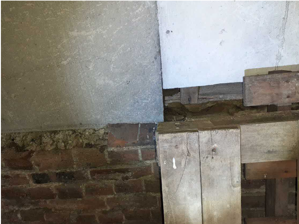
Photograph 38: Gap leading to cavity in interior of Building 2
