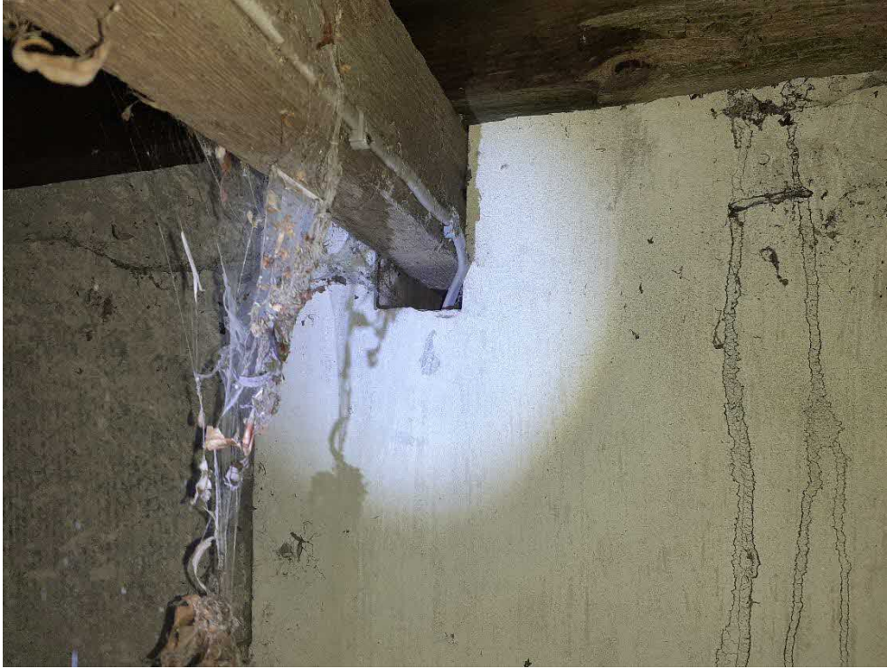
Photograph 37: Gap leading to cavity in interior of Building 2
