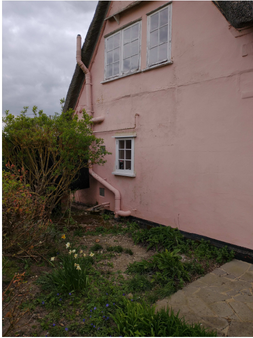
Figures 11.1 – upvc soil and vent pipe to be removed – also note numerous areas of modern render repairs with would be made good and restored with new lime render on lathes (see section 13 for lime render proposals)
