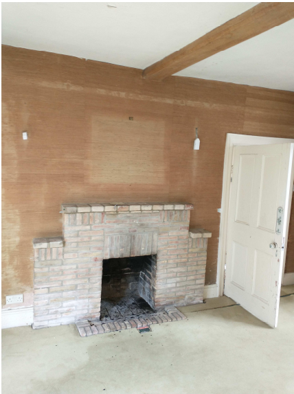
Figures 3.1 – drawing room modern fireplace surround to be removed (for re-fitting of existing Aga)
