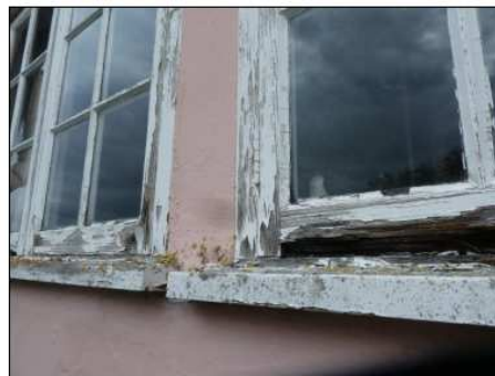
Rot to stairwell window
