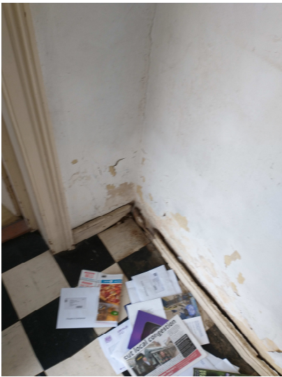
Figures 4.3 – decaying floor in the lobby to be investigated, rot treated/timbers replaced as necessary, and additional sub-floor ventilation provided. (Also see Design & Access Statement fig 1.2.2 for photo of drawing room floor with water damage)
