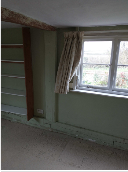
Figures 4.2 – sitting room with concrete floor (just visible through fraying carpet edges) – also showing previous timber frame sole plate repairs which were carried out when this area was underpinned
