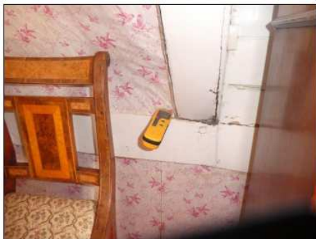
Seepage to base of dormer in bedroom 1
