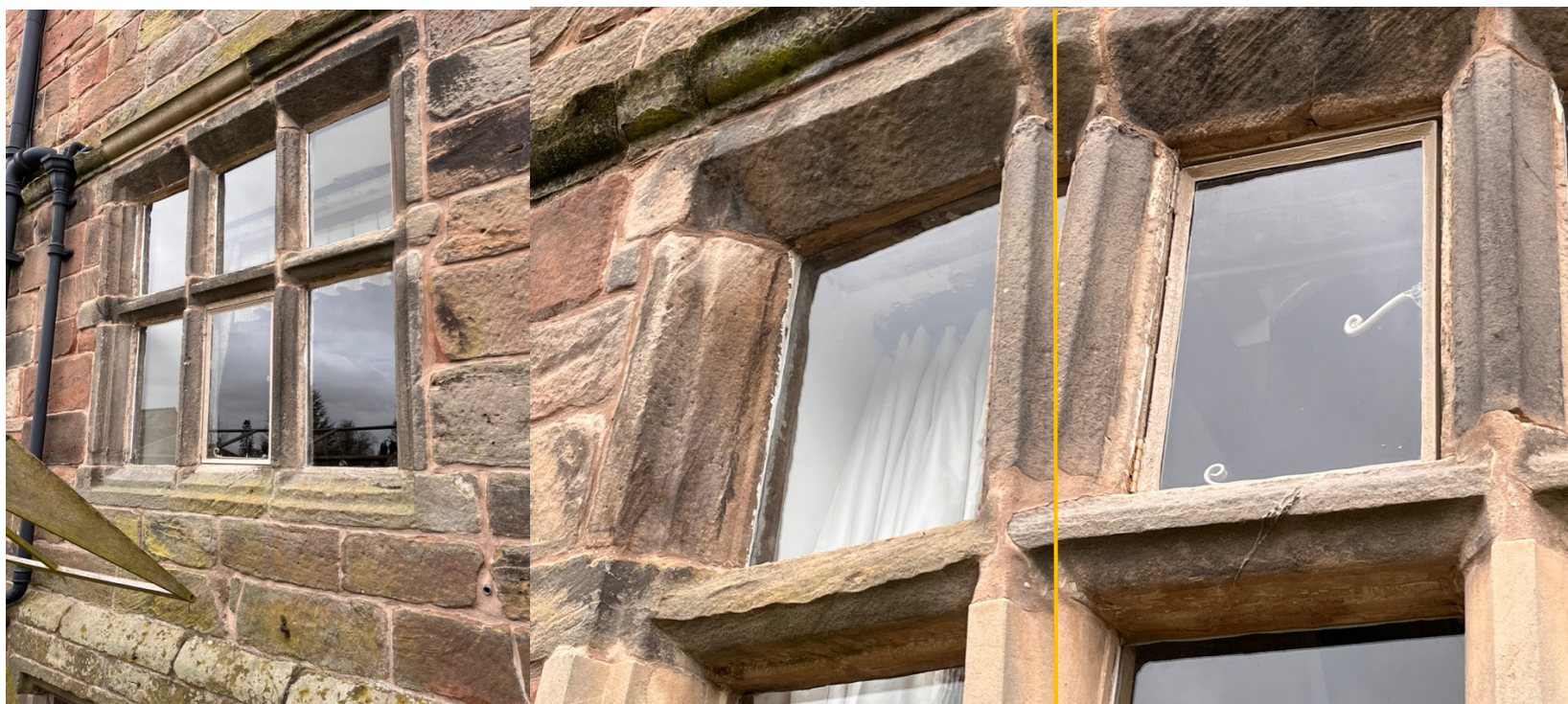
Fig 5. Top. Window photographs March 2023. Note silicon and historic cementitious repair.
