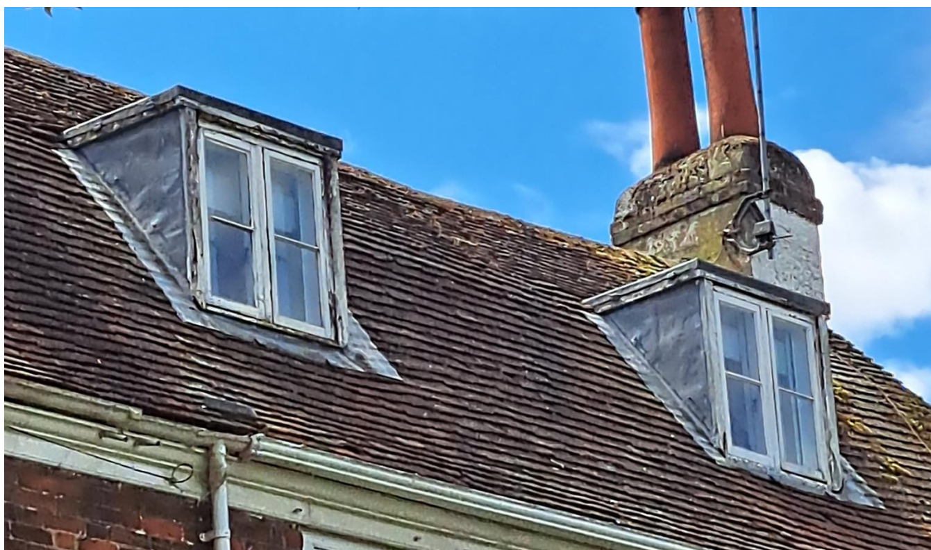
View of second floor dormers from front of house. Dormer to left hand side is hereon referred to as LHD1 and dormer to right hand side RHD2.
