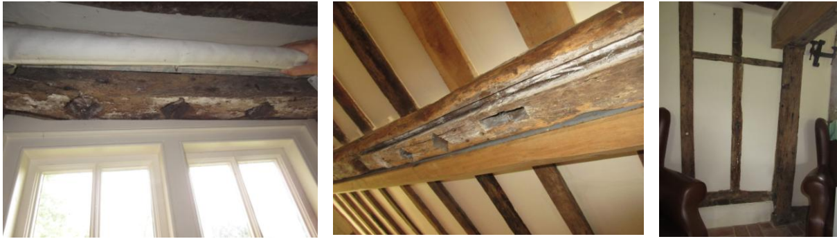
Left: diamond mullion mortices in underside of window lintel in NE wall; Centre: underside of re-used cross axial beam with mullion mortices, shutter groove and rectangular mortice for stud, reinforced with modern oak beam on SE face; Right: former doorway in SW wall
