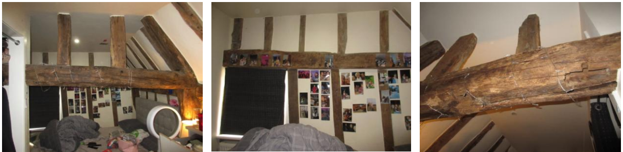
Bedroom 3: Left: looking SE showing open studs above tie beam; Centre: SE end wall with window beyond tie beam; Right: shutter groove and mullion mortices in underside of tie beam
