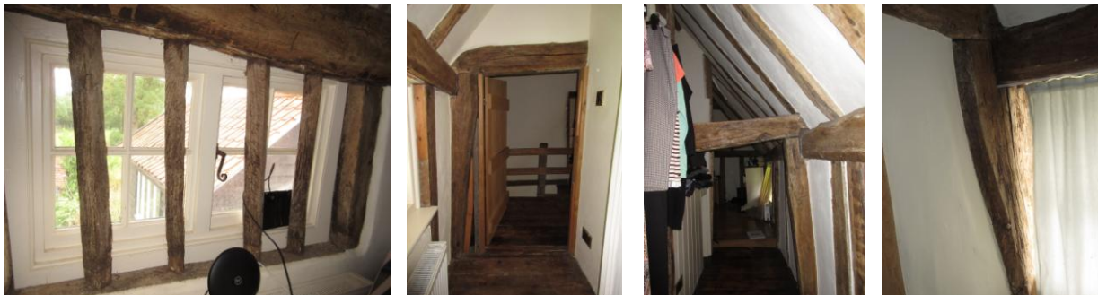
Left to Right: detail of diamond mullion window with shutter groove; Looking SE showing jowelled main post between passage and landing; Looking NW down passage to bedroom 1 showing tie beam on SE side of stack; jowelled main post in SW corner of bedroom 2
