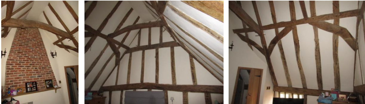
Left: looking SE showing exposed brickwork of stack and cambered collar of clasped purlin roof; Centre: looking NW showing exposed studs, tiebeam, common rafters, collar and cranked windbrace; Right: SW roof slope showing pairs of cranked windbraces and top of mullion window, door leads to shower room beside stack
