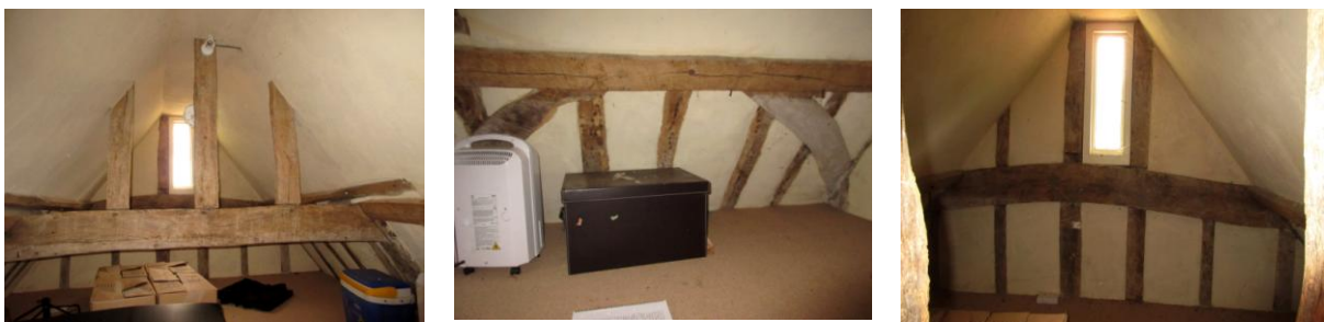
Left: looking SE showing open studs above collar; Centre: arched windbraces in NE roof slope; Right: window inserted between studs in SE gable
