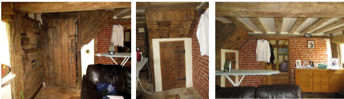
Left: looking SE showing door to stairs, front door on left; Centre: looking NE, showing door to understair cupboard; Right: looking SE showing brick partition wall & door to dining room
