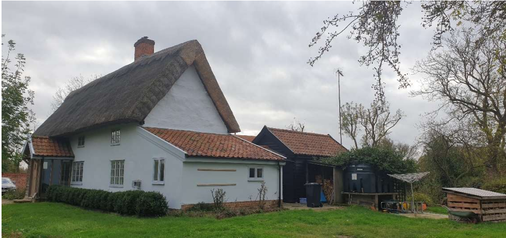
View of the northern gable, with replacement lean-to, and converted building beyond (black clad), plus lean-to log store and oil tank
