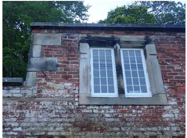
Crevices present in the brick work
