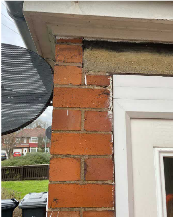
Photograph 15. External Wall to Porch Leaning Out
