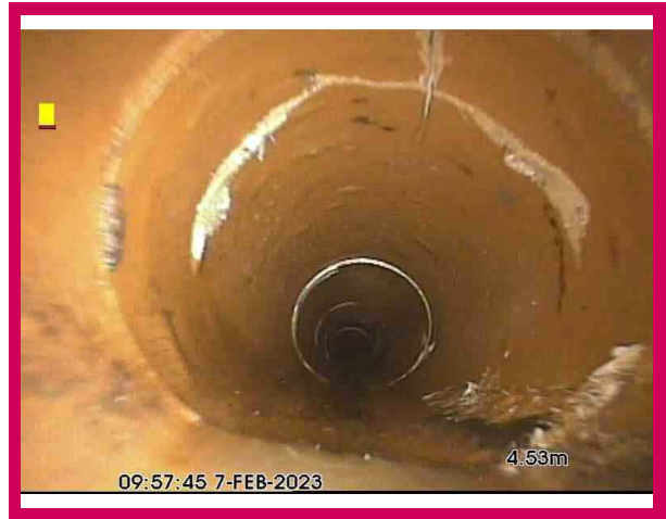
2, 00:00:19, 4.53 m Fracture, circumferential at joint from 12 o'clock to 12 o'clock
