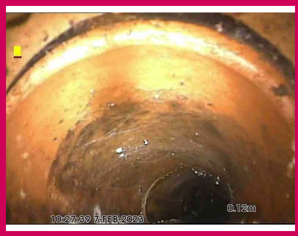
1, 00:00:05, 0.14 m Joint displaced, medium
