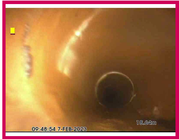
2, 00:00:58, 13.54 m Crack, circumferential at joint from 12 o'clock to 12 o'clock
