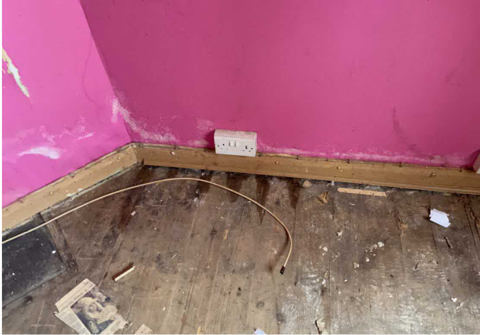
Photograph 13. Ground Floor Bedroom Showing Water Ingress
