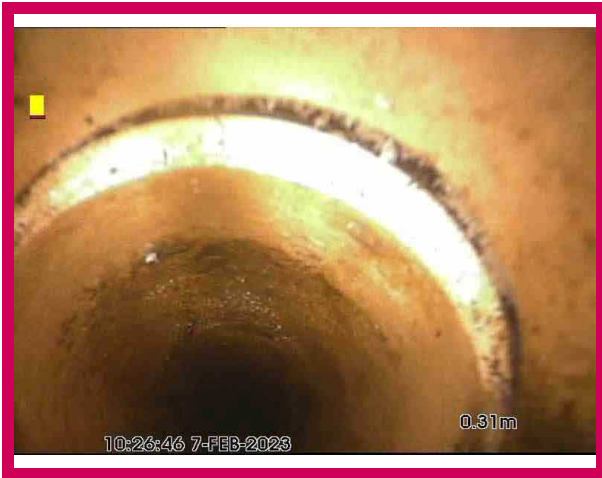
1, 00:00:13, 0.40 m Joint displaced, medium
