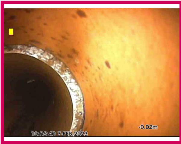
1, 00:00:03, 0.10 m Joint displaced, medium
