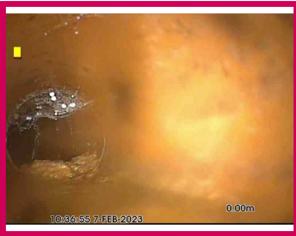
1, 00:00:05, 0.30 m Attached deposits, fouling from 4 o'clock to 7 o'clock, 10% cross-sectional area loss
