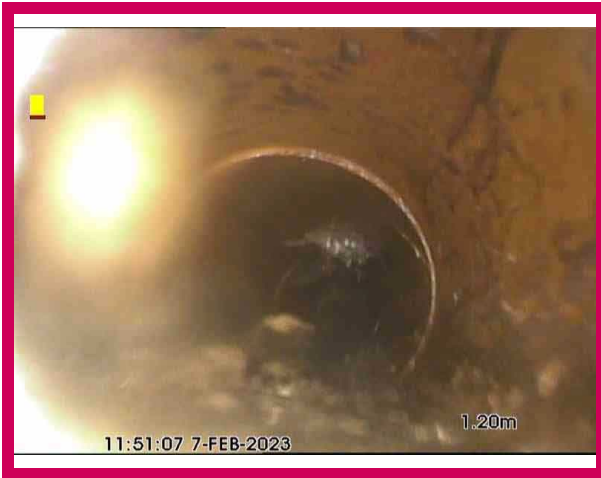
1, 00:00:05, 1.27 m Attached deposits, encrustation from 3 o'clock to 7 o'clock, 10% cross-sectional area loss, start
