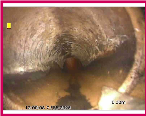
1, 00:00:06, 0.33 m Joint displaced, medium
