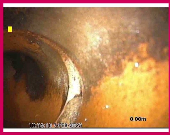
1, 00:00:03, 0.20 m Joint displaced, medium
