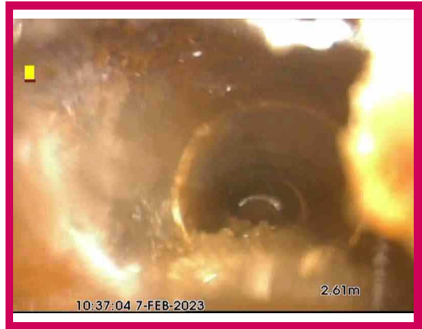
2, 00:00:15, 2.61 m Attached deposits, fouling from 4 o'clock to 7 o'clock, 20% cross-sectional area loss
