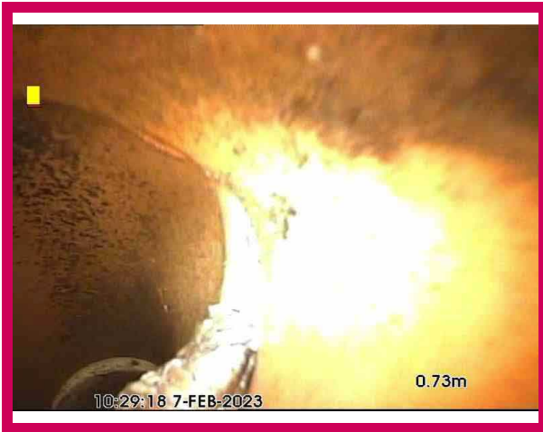
1, 00:00:10, 0.73 m Joint displaced, medium
