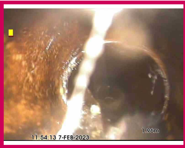
1, 00:00:11, 0.00 m Attached deposits, fouling from 3 o'clock to 8 o'clock, 15% cross-sectional area loss, start
