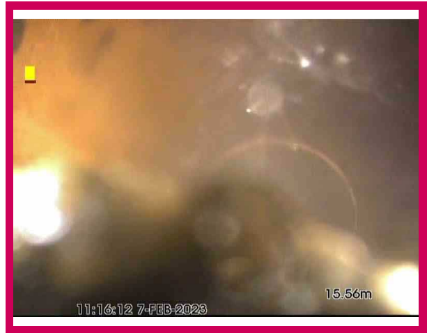
2, 00:01:01, 15.56 m Attached deposits, fouling from 3 o'clock to 9 o'clock, 20% cross-sectional area loss
