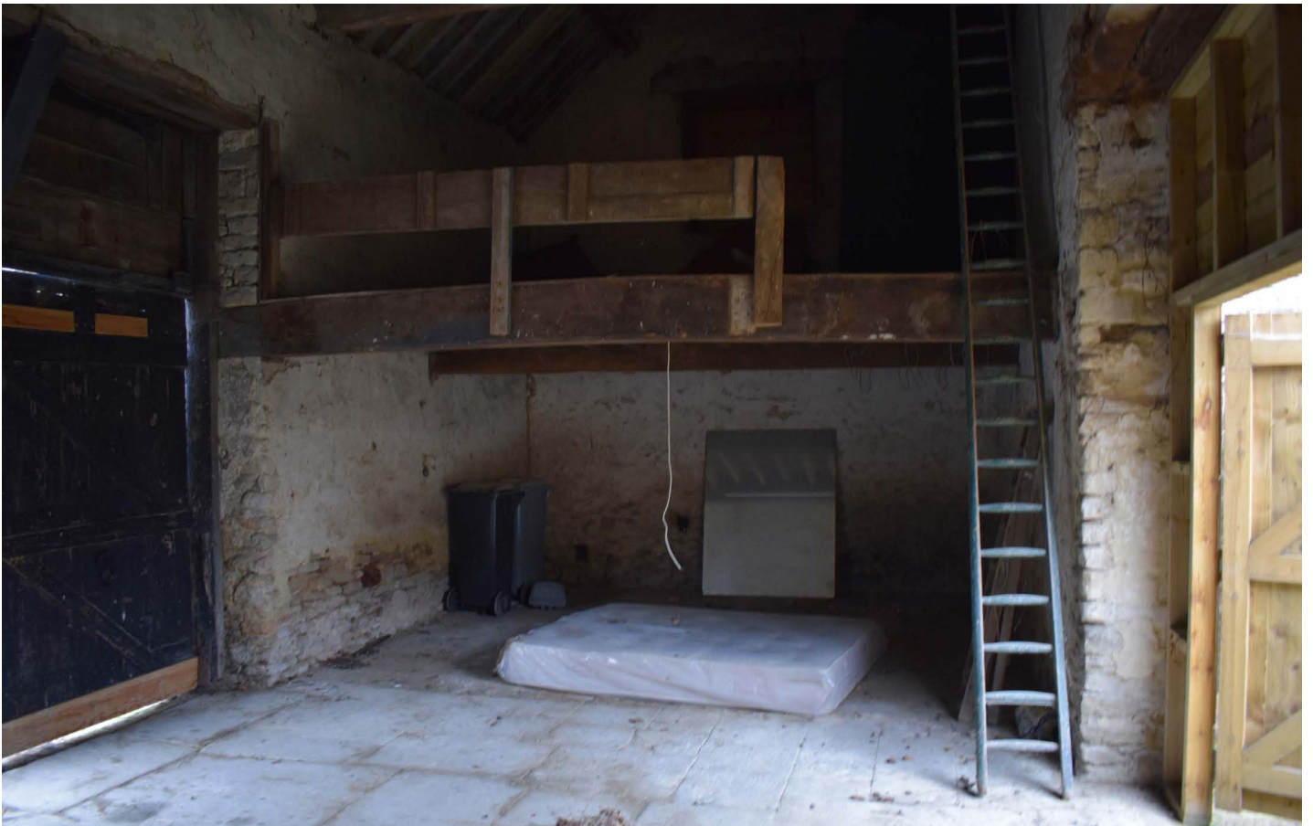
View looking north to hay loft with door to Queen Street to the left and garden to the right with a stone slab threshing floor
