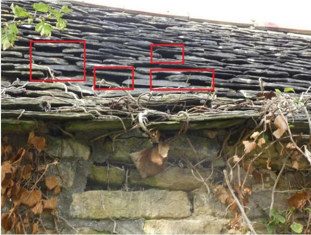
Photos 13 and 14 – Gaps under roof slates and clay ridge tiles
