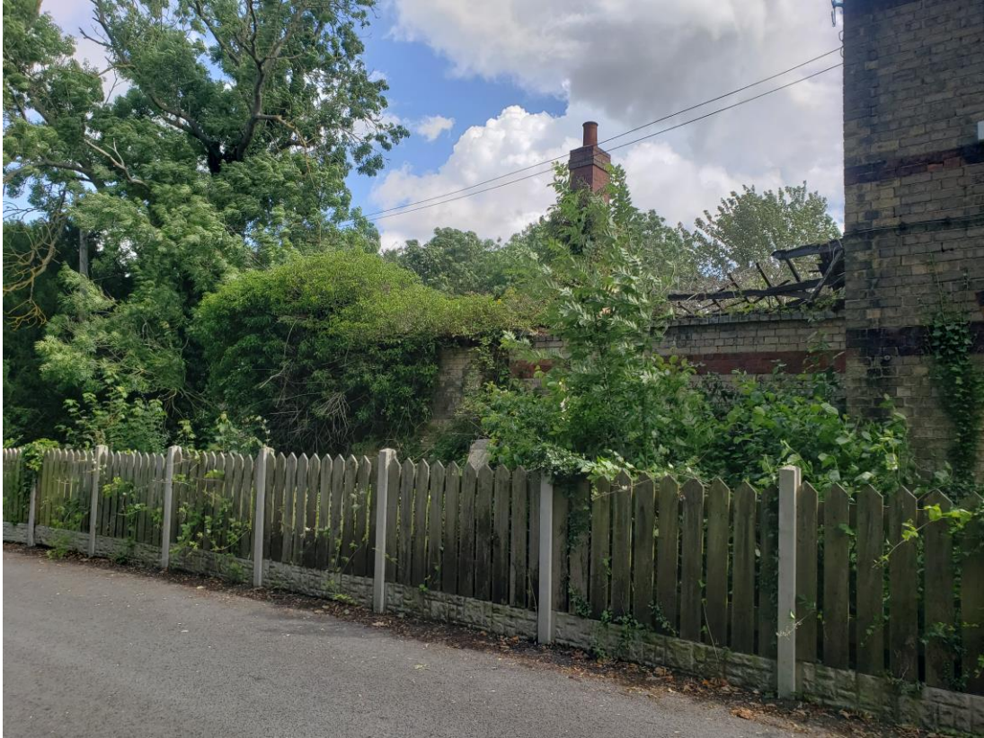
Image above showing the collapsed roof over Outbuilding 1 and the overgrown garden / outbuilding 2 and 3
