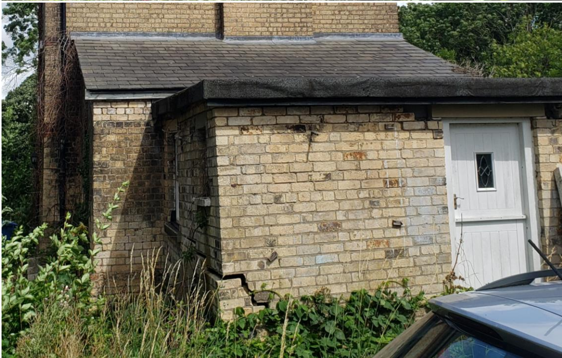
2 images above showing subsidence in the kitchen (South West Corner)
