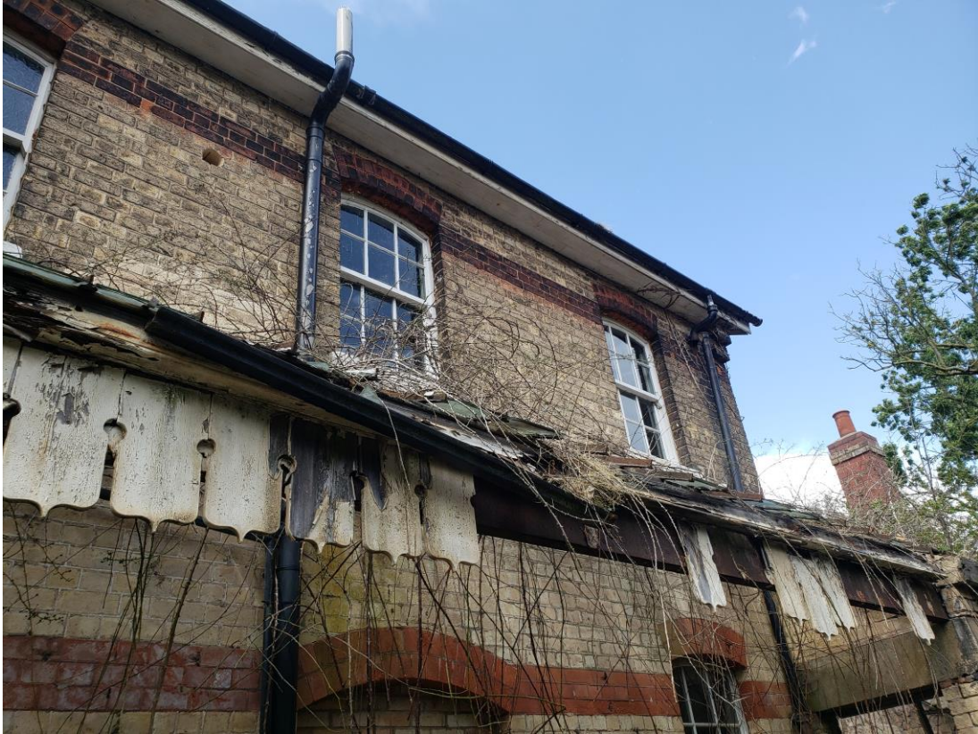
Image above shown the glazed canopy and timber feature fascia in dis-repair
