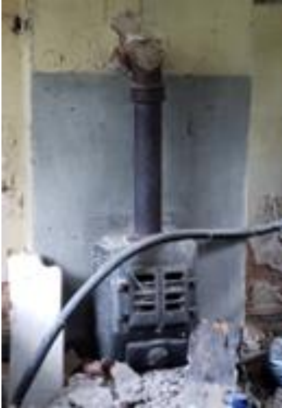
Fire place 3 in Waiting area
