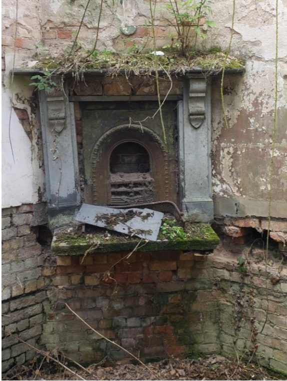
Fire place 5 in Outbuilding 1 (floor missing)
