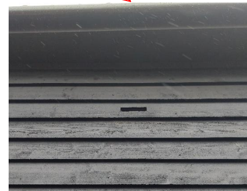
Access to the bat boxes cut into the weather boarding. The holes can be cut by scalloping the underside of the board where it covered the board below to reduce water ingress.
