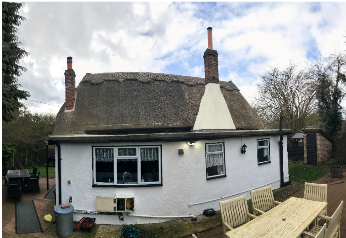
b - East corner showing rear elevation of property and the dilapidated stores in the background
